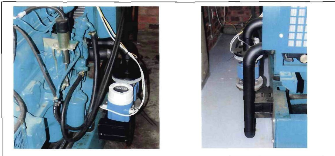
Figure 23: Radiator flow meter installation position
