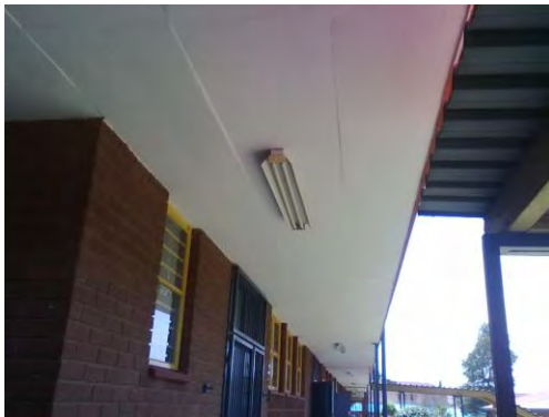
Figure 4.4: Lighting of School
