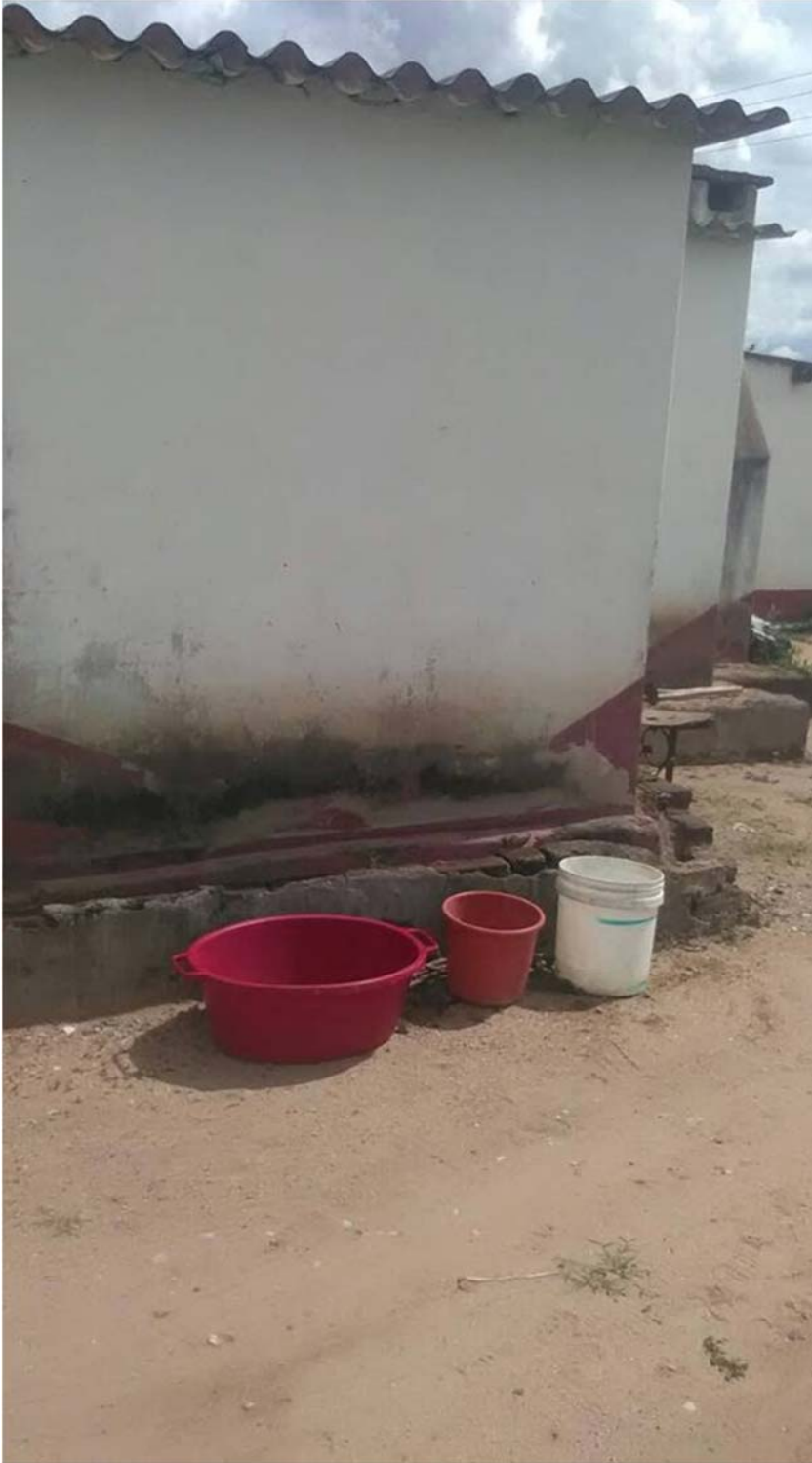
Image 6.2: Rooftop water-harvesting technique used in Chivi
