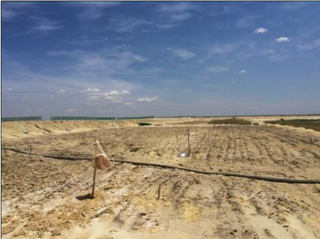
Figure 3.14: Top-flat trial plots on the Crown gold TSF after lime and compost were applied and ripped into the tailings surface. Photo taken by C.A. Kruger, 4/3/2016.
