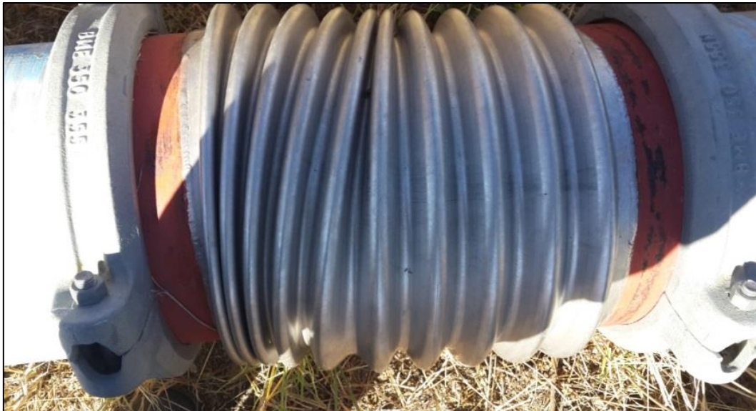
Figure 75: Impact of temperature change on the compressed air pipe network in Case Study 1
