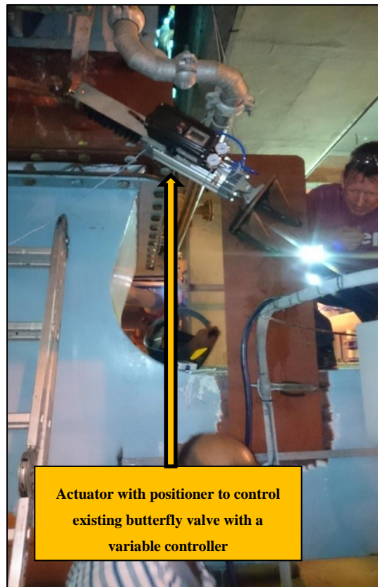
Figure 85: Installing an actuator on an existing butterfly valve for improved throttle control
