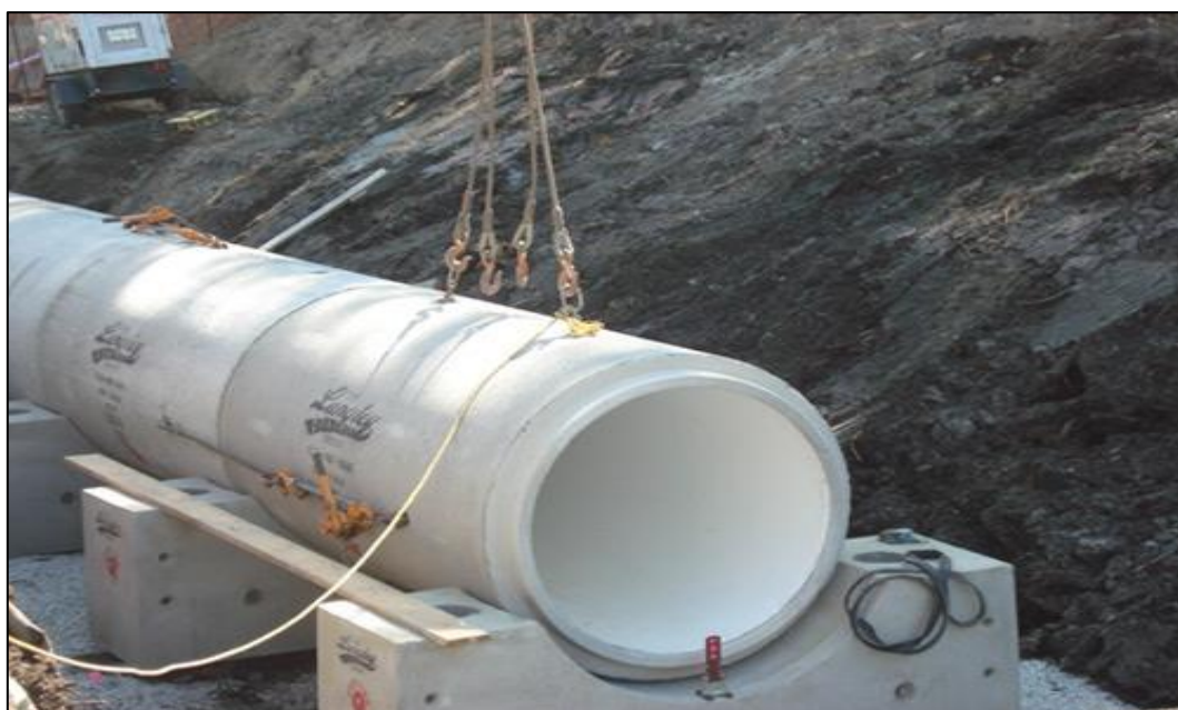
Figure 71: Concrete pipe support for reliable support
