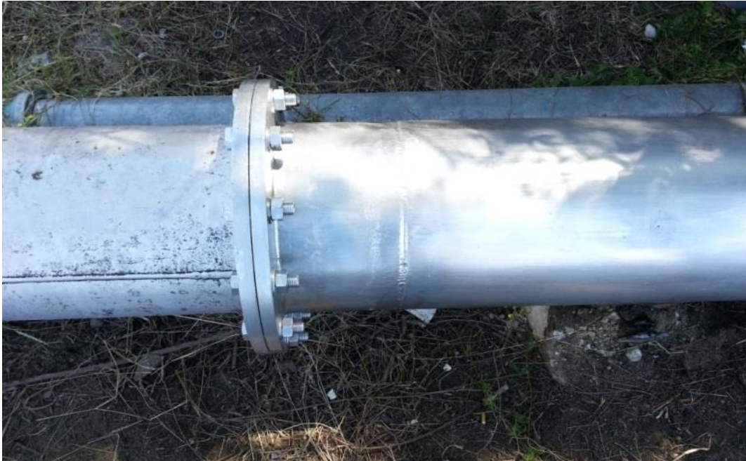
Figure 74: Repaired flange connection on the compressed air pipe network of Case Study 1
