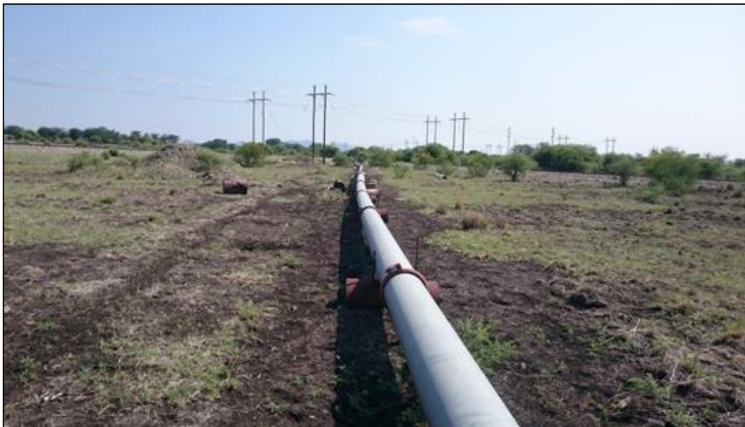
Figure 69: Pipeline of compressed air system connecting main shafts and compressors
