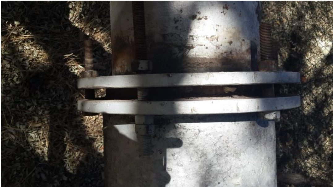
Figure 73: Poor pipe connection on the compressed air network of Case Study 1
