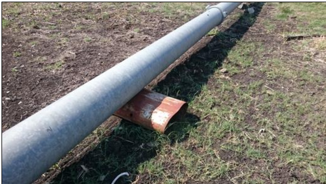
Figure 70: Collapsed pipe support in Case Study 1
