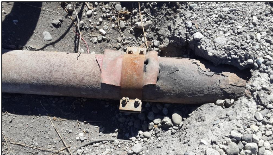
Figure 79: Improper leak repair method on the compressed air pipe network of Case Study 1
