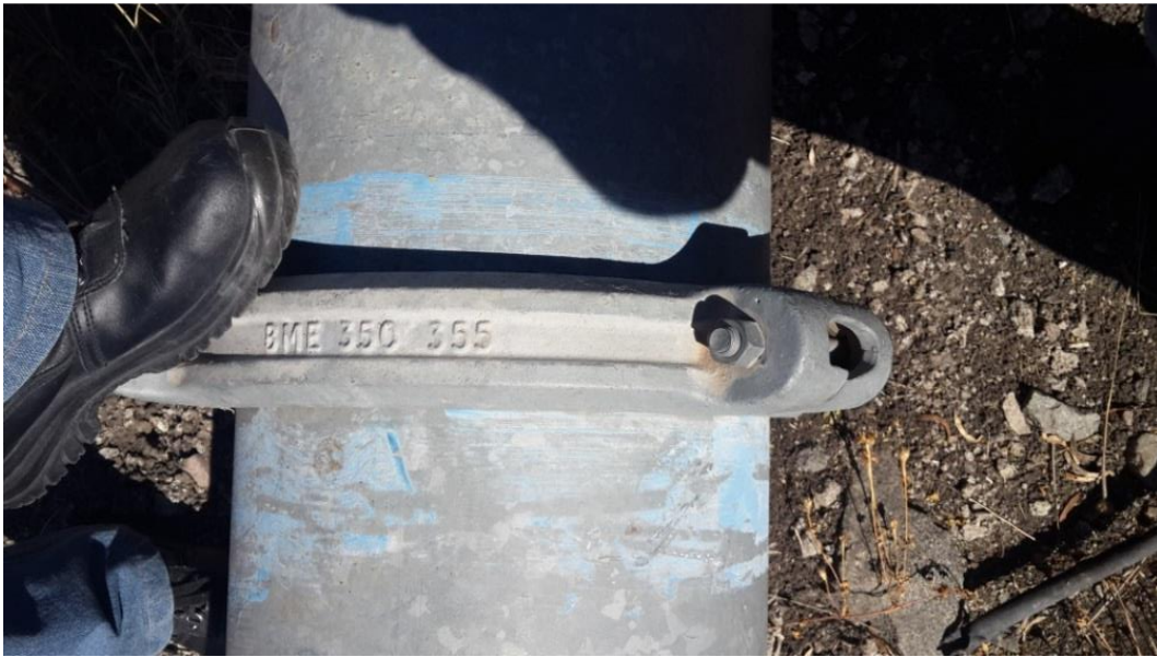
Figure 72: Victaulic joints connecting pipes in Case Study 1
