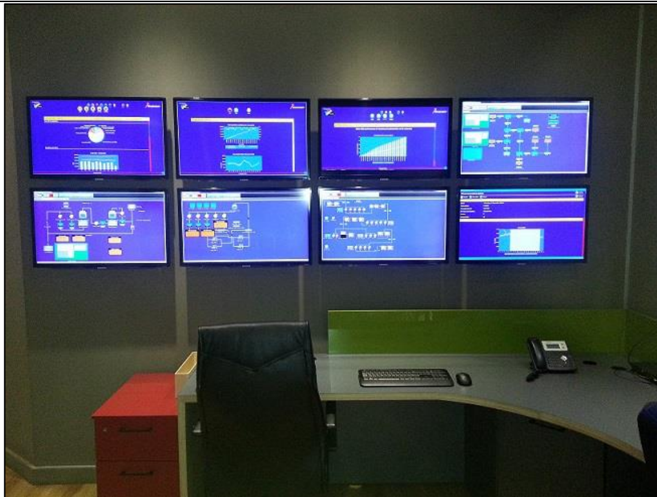
Figure 64: ESCO control room
