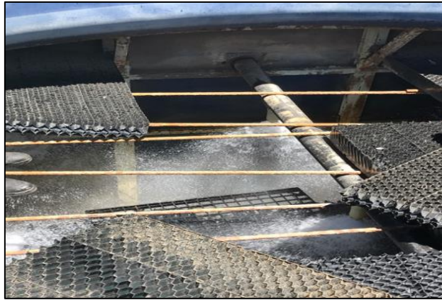
Figure 28: Mine A drift eliminators 17
