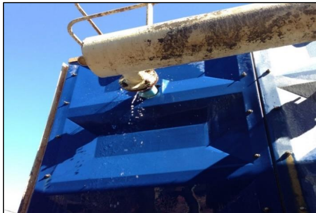
Figure 29: Mine A pipework 18
