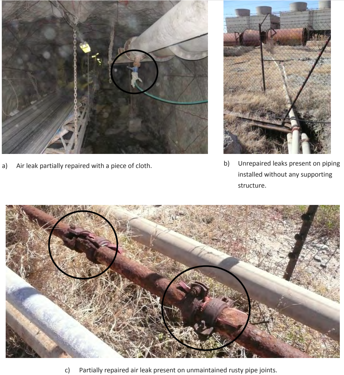
Figure 2.13 – Typical unmaintained piping sections.
