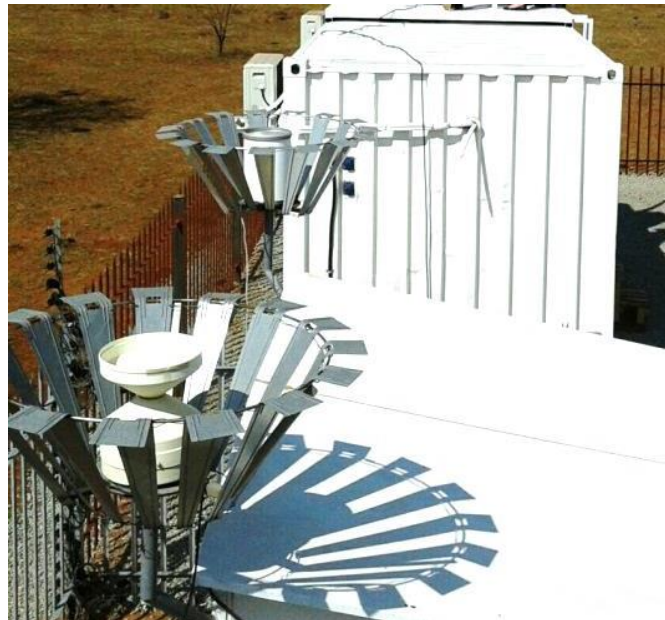
Figure 3.8 The Vaisala QMR102 and Casella 0.1 mm tipping bucket rain intensity instruments as installed at the Welgegund measurement station (Photo credit: Dr. M. Josipovic).
