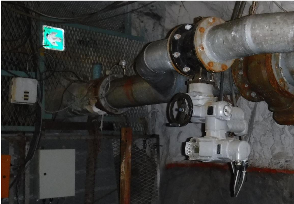
Figure 36: New control valve set-up
