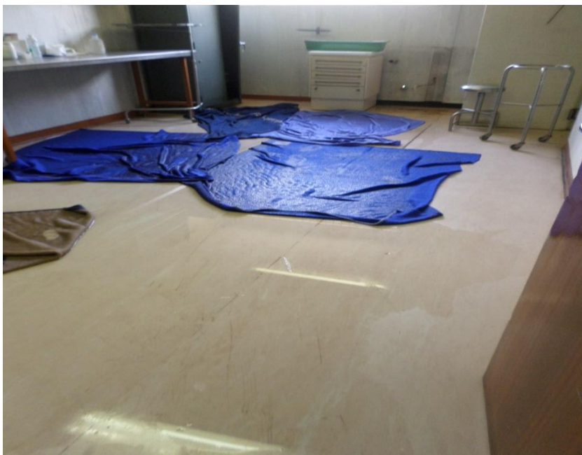
Figure 7: Flooding of the room resulting from a leaking pipe (Zola CHC, 2014)
