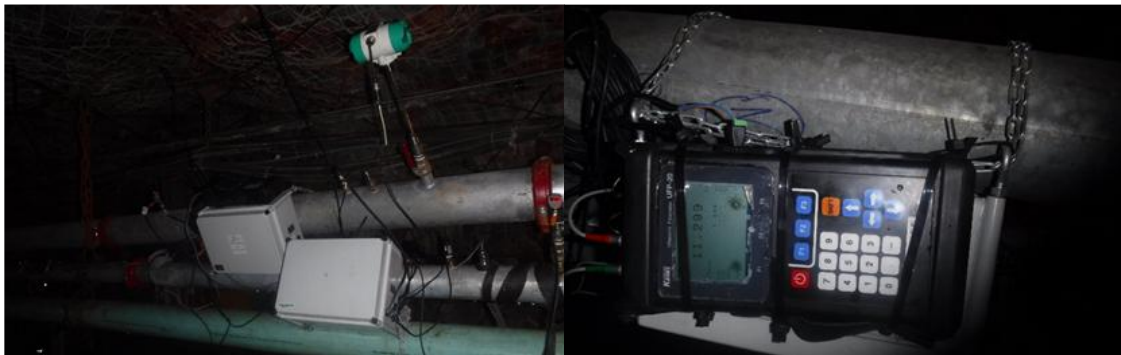
Figure 38: Pictures of portable ultrasonic flow meter setup (picture taken by author).
