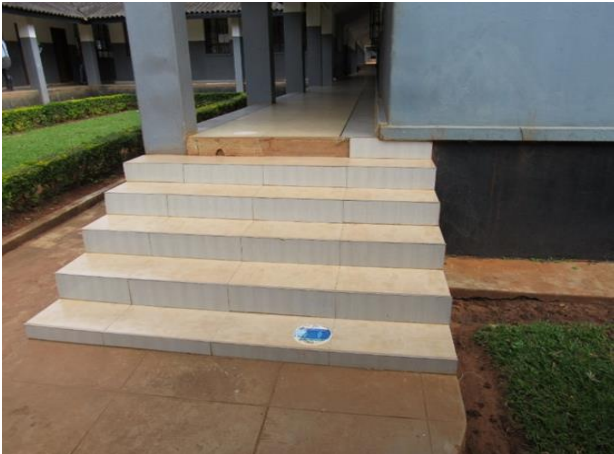
Figure 5-5: Steep stairs at Chalimbana University (Source: Researcher's archive, 2022/2023)
