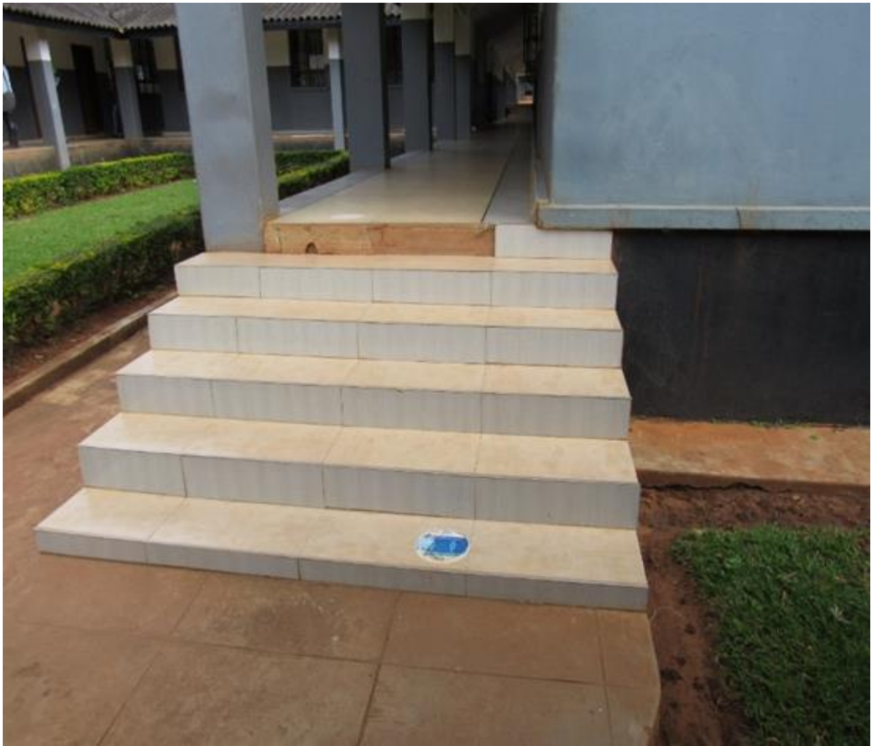
Figure 6-4: Staircase with no guard rail at Chalimbana University (Source: Researcher's archive, 2022/2023)
