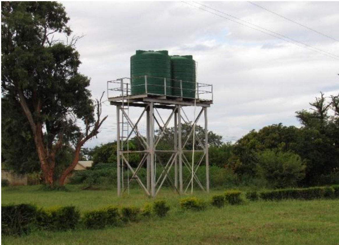
Figure 6-10: Overhead storage water tanks at Chalimbana University (Source: Researcher's archive, 2022/2023)
