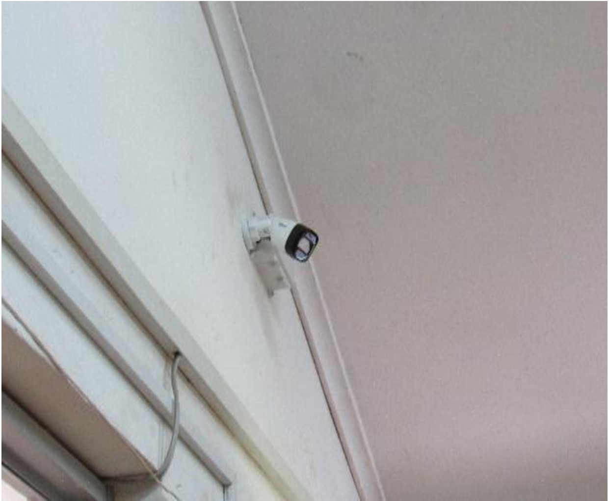
Figure 6-2: CCTV at Chalimbana University (Source: Researcher's archive , 2022/2023)
