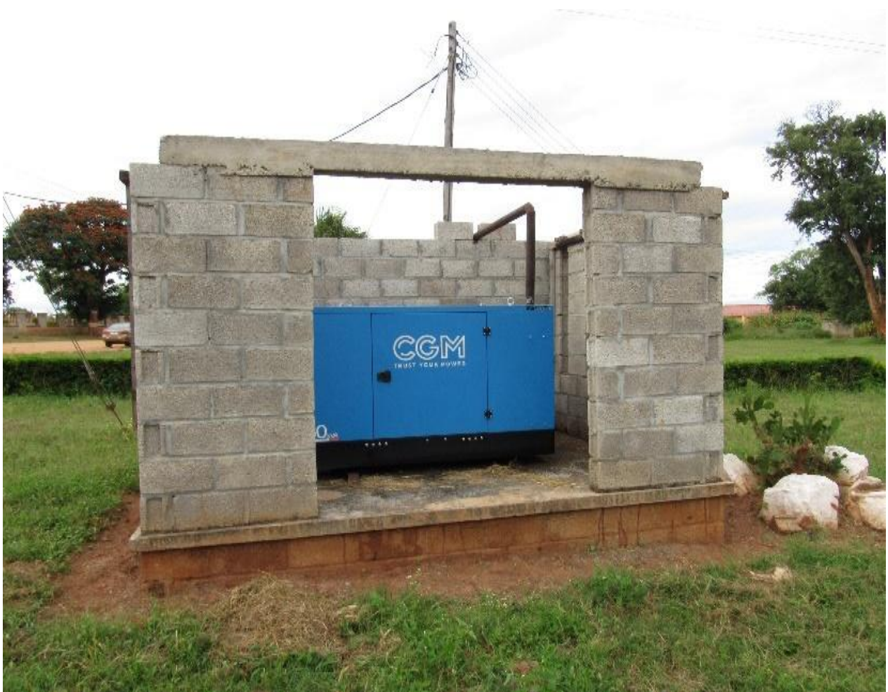
Figure 5-11: Poorly secured generator at Chalimbana University (Source: Researcher's archive, 2022/2023)
