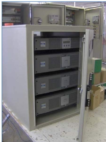
Figure 33: UPS to be installed
