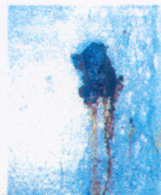
Coating failure resulting in corrosion of underlying steel.
