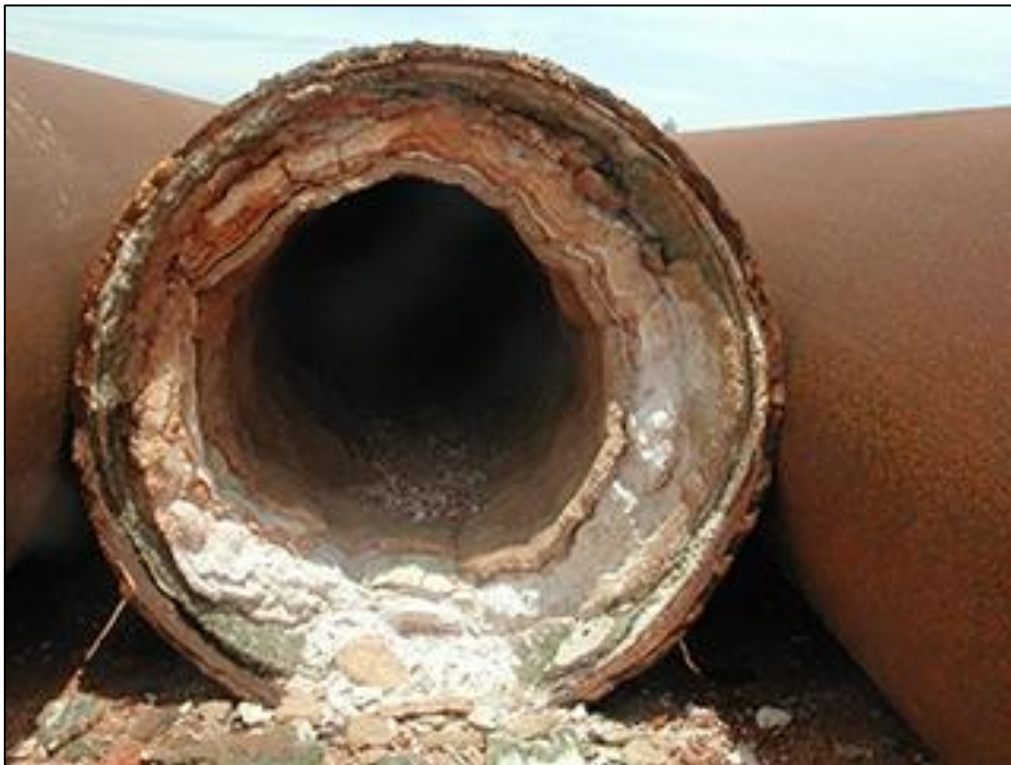
Figure 2.15: Scale build-up within a pipe (Envirofluid, 2014)
