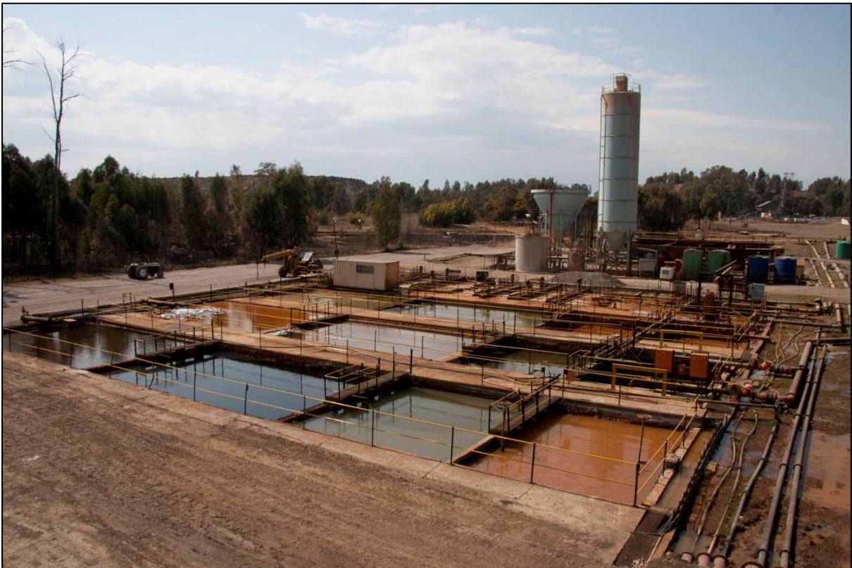
Figure 2.11: Harmony gold mining company's Tweelopiespruit AMD treatment site (Waanders, 2015)
