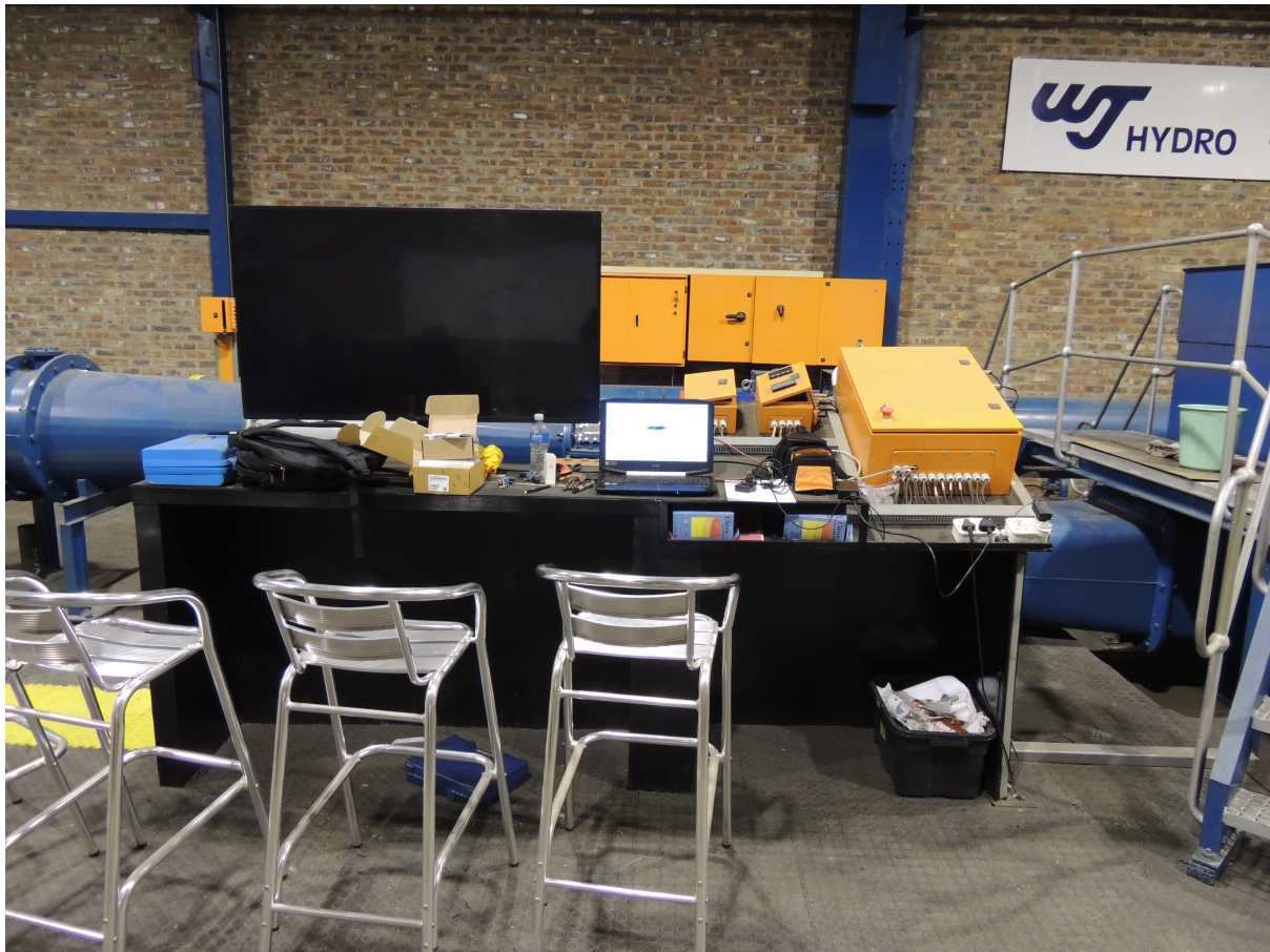
Figure 4.30. IFM PLC and data logger installed at WJ Engineering
