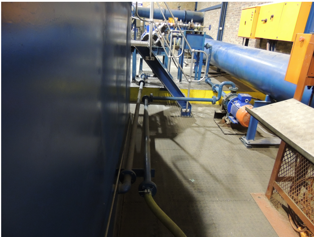
Figure 5.8. Cooling cycle pipework running adjacent to water tank
