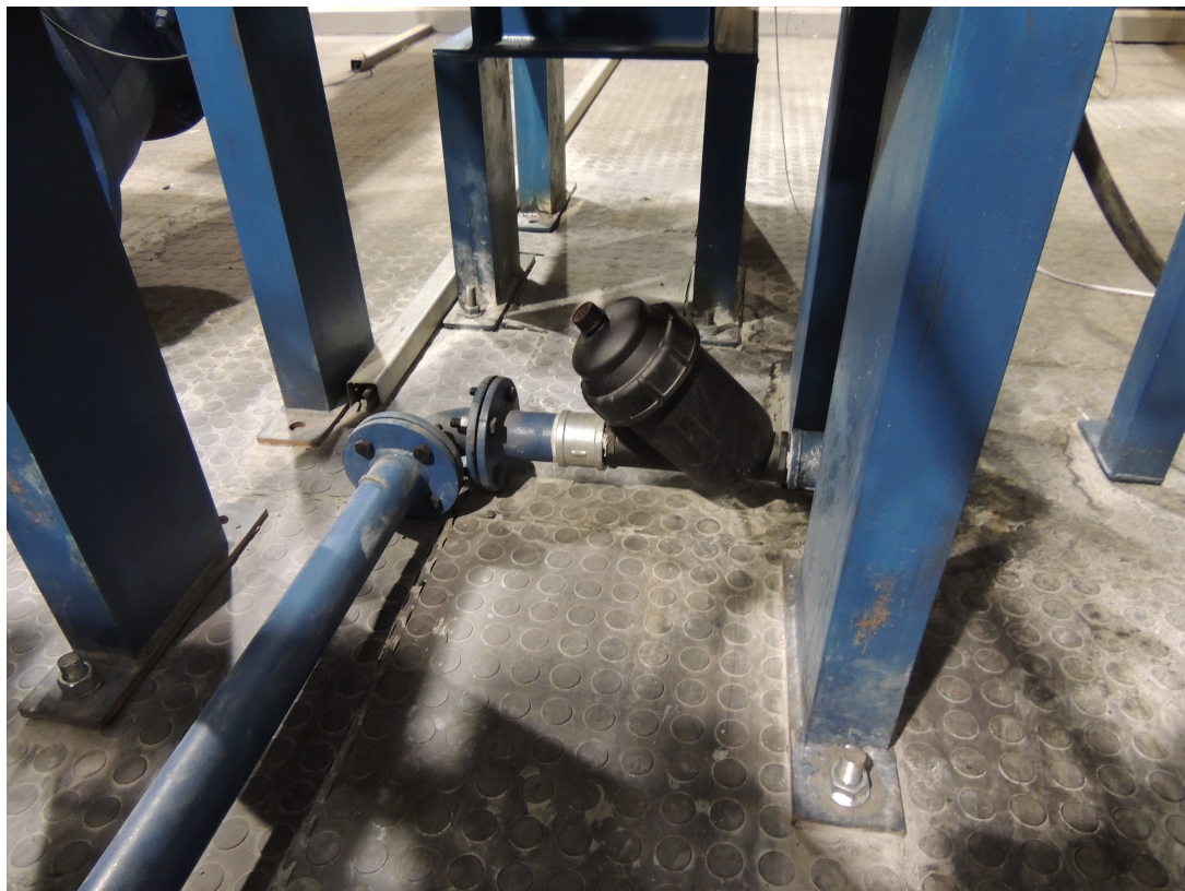
Figure 5.10. Inline filter to clean inlet water
