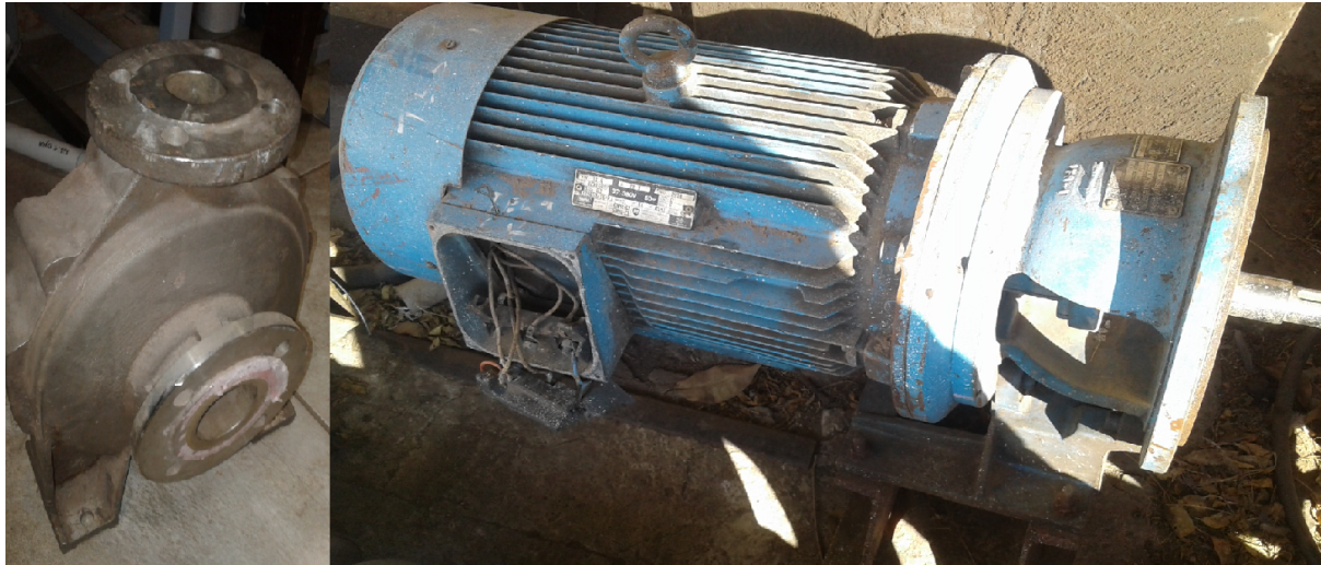
Figure 4.25. Rapid Allweiler CLT40-250 centrifugal pump before refurbishment
