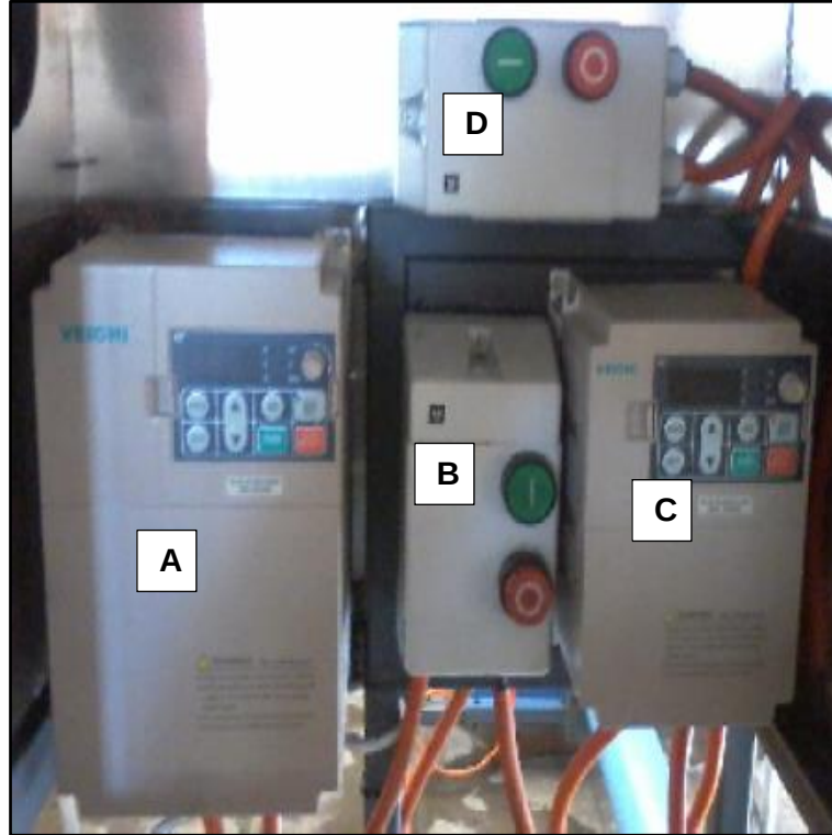
Figure 3.7: Control unit for the centrifugal fan and vibration motor
