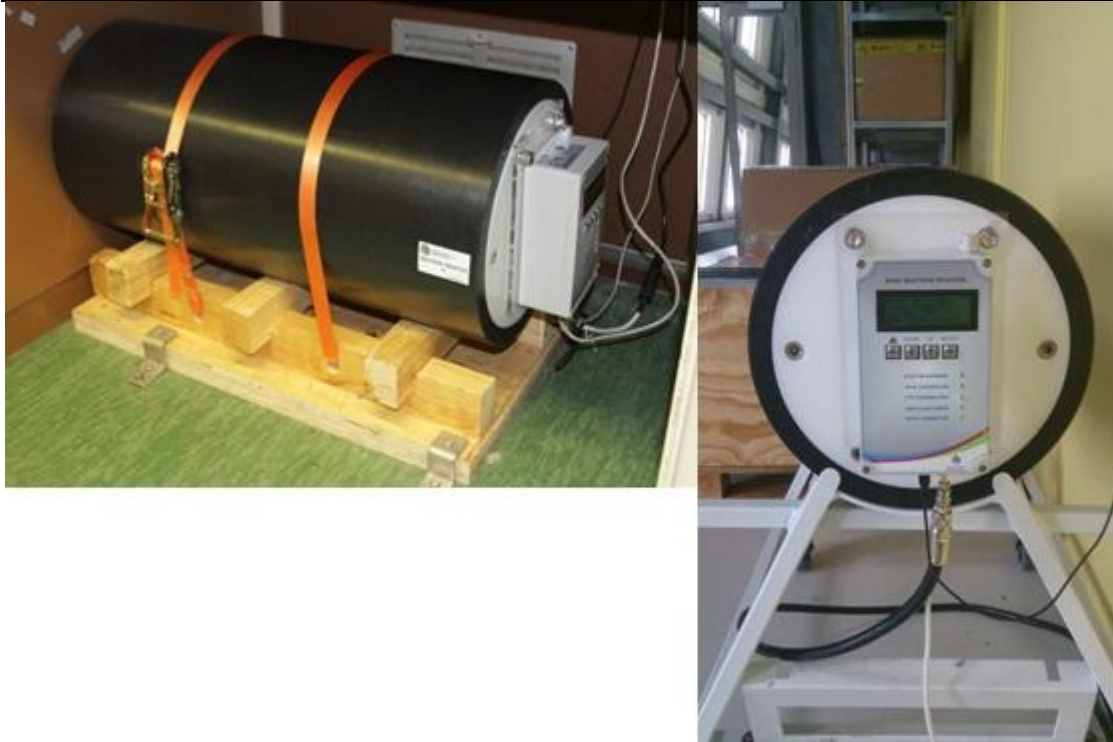
Figure 4-33: ADM (a) Polarstern and (b) Neumayer installations
