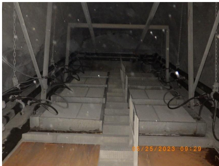
Figure 8: Cooling-coil BAC (Personal Picture)
