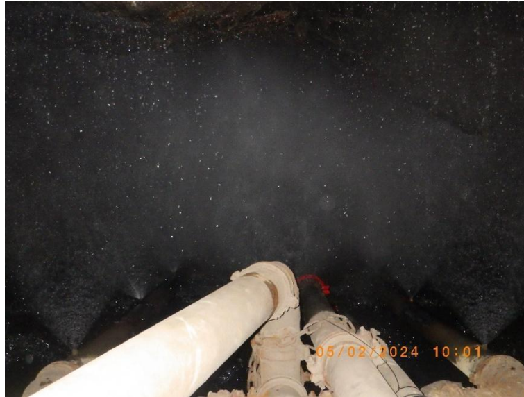
Figure 7: Horizontal force-draft BAC (Personal Picture)
