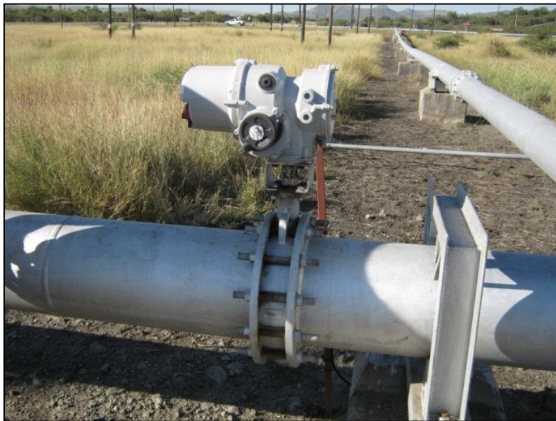
Figure 20: Example of a surface control valve 9
