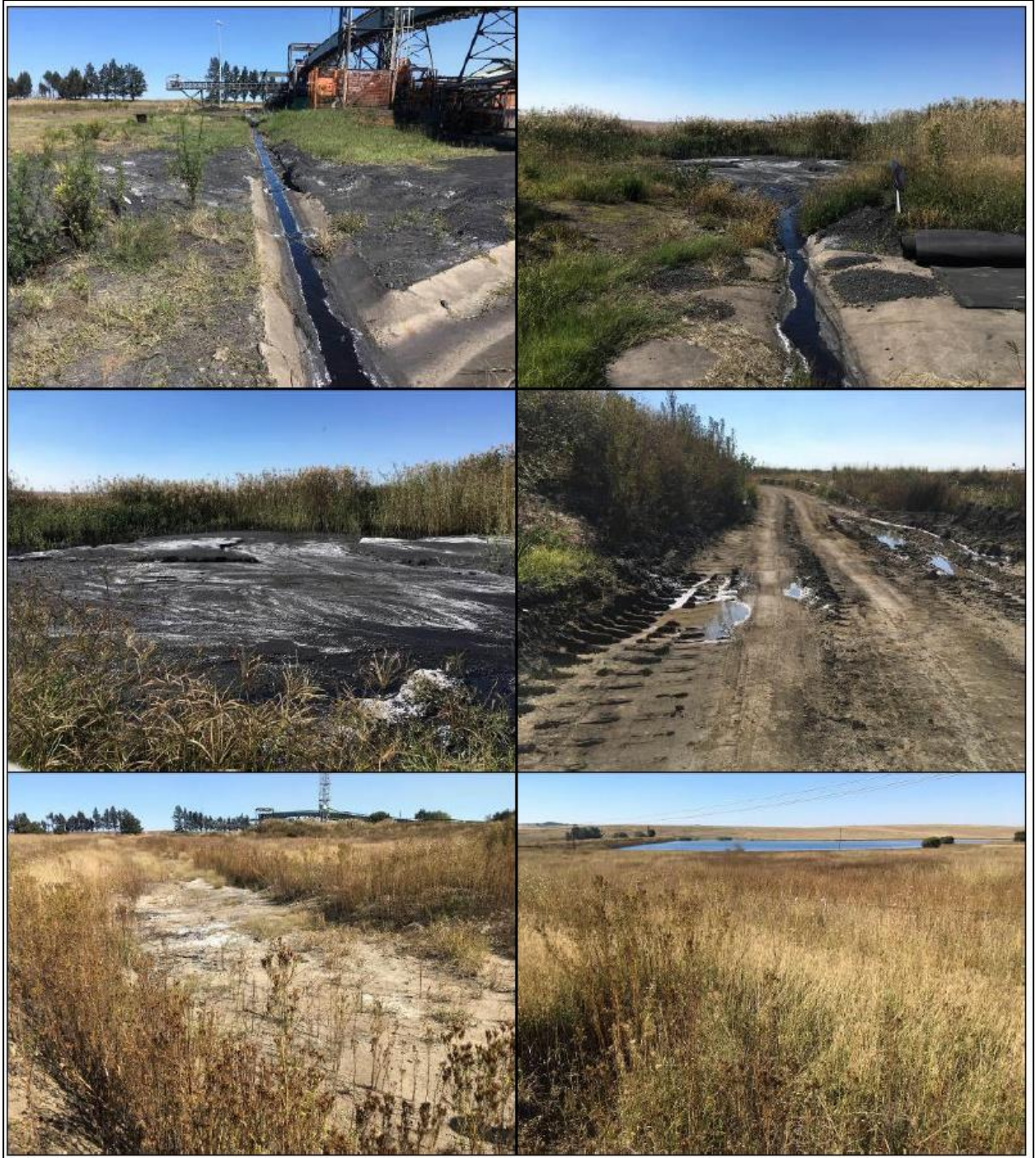
Figure 2-1: (Top left): Main inflow channel from the conveyor system to the overland sump. (Top right): View of the inflow channel into the overland sump showing coal fines and sediment buildup. (Middle left): Close-up of sediment accumulation in the sump. (Middle right): Seepage visible below the wall of the overland sump. (Bottom left): White residue on the soil about 100 meters downslope from the overland sump. (Bottom Right) View of the Krapfontein clean water dam, located around 330 meters downslope from the overland sump. (Source: Wetland Consulting Services (Pty) Ltd., 2019)
