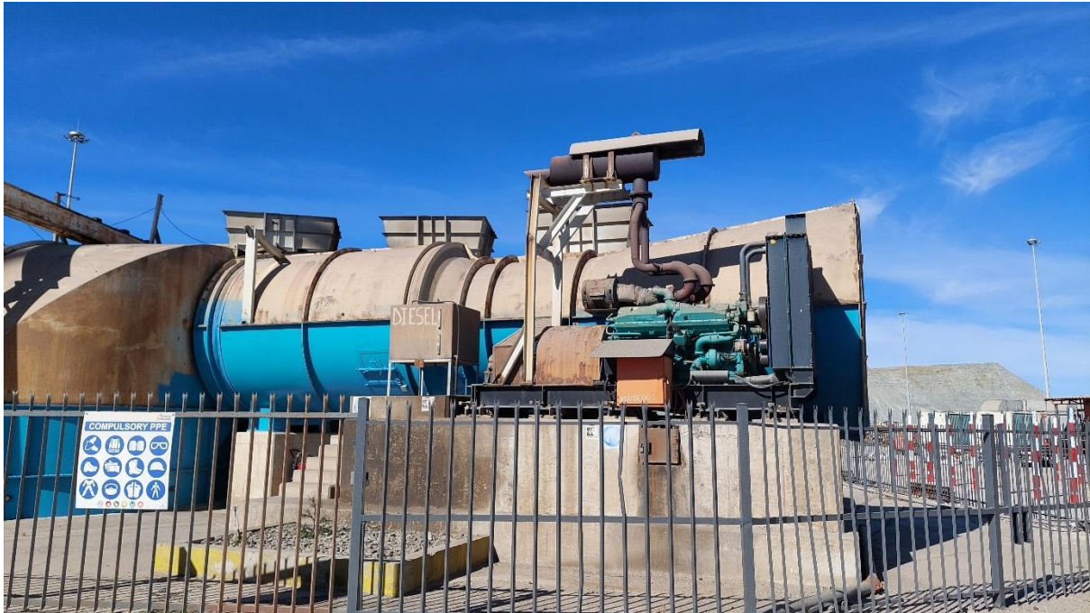
Figure: Emergency diesel-powered axial surface fan 3
