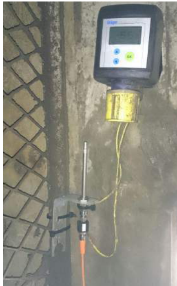
Figure 3.3: BAC outlet temperature sensor
