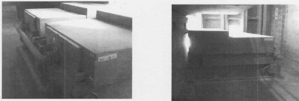
Figure 28: Soft starters installed on the factory .
