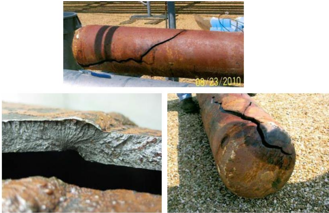
Figure 1-3: Failed 12" pipe at the Theodore, AL Millard refrigeration plant [9].
