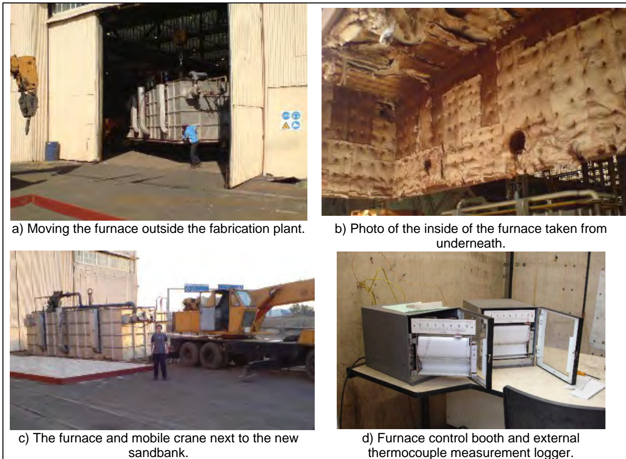
Figure 5.4: Preparing the furnace for the nitriding plant.
