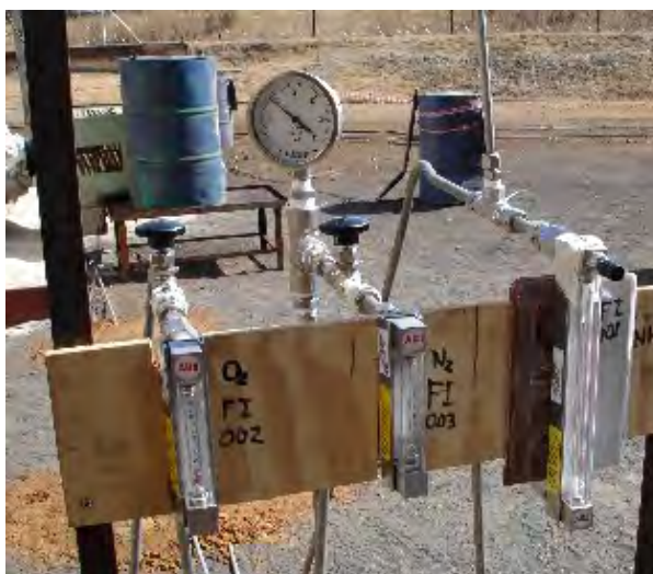
Figure 5.10: The Gas Supply PFM Control station.
