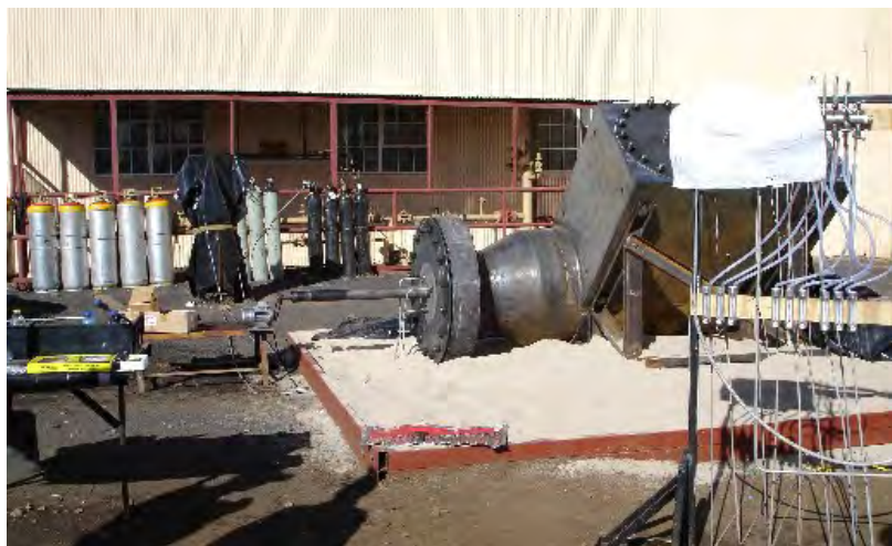
Figure 5.6: A landscape photo of the plant before the Top Hat was lowered over the CUD.
