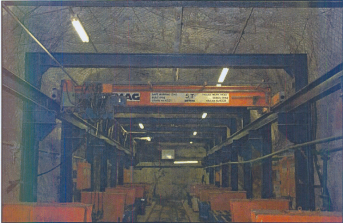
Figure 37: Photo of a typical battery bay
