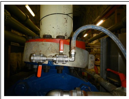
Figure B-11: Discharge pressure sensor
