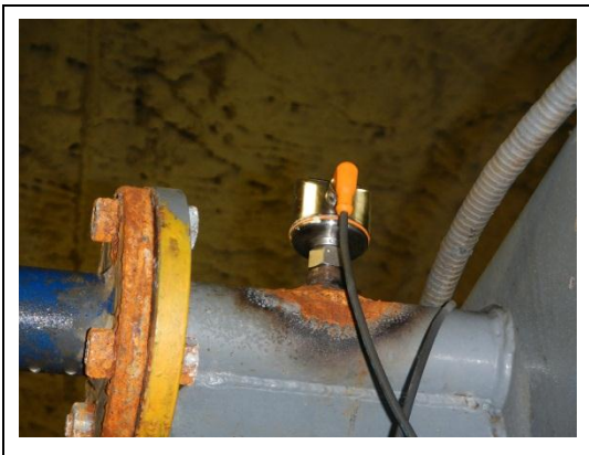
Figure B-5: Motor cooling water flow switch
