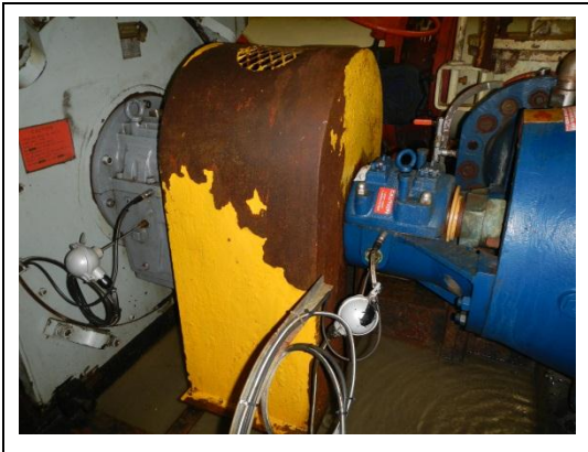
Figure B-21: Motor and pump coupling
