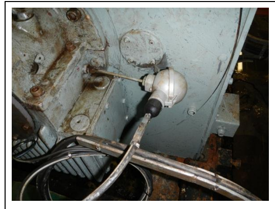
Figure B-10: Motor NDE temperature sensor
