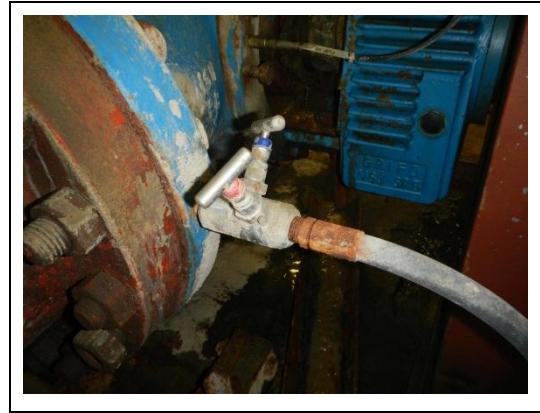
Figure B-2: Suction pressure switch
