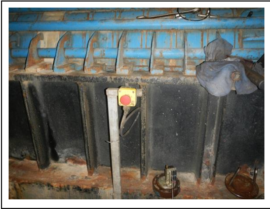
Figure B-1: Emergency switch
