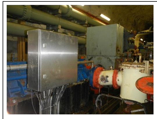
Figure B-6: Instrumentation junction box
