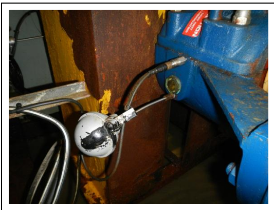
Figure B-23: Pump DE temperature probe and vibration sensor
