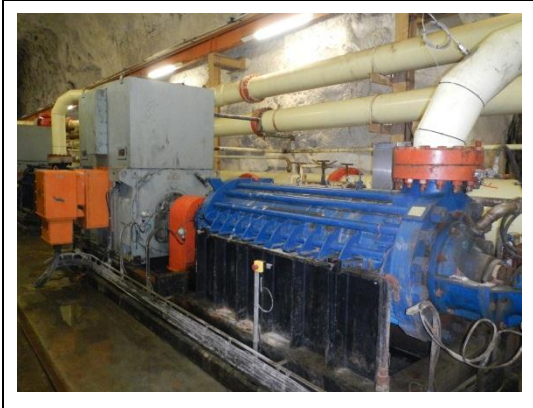
Figure B-7: Pump and motor
