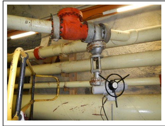
Figure B-16: Discharge NRV and actuated gate valve
