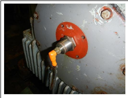
Figure B-9: Motor shaft displacement sensor
