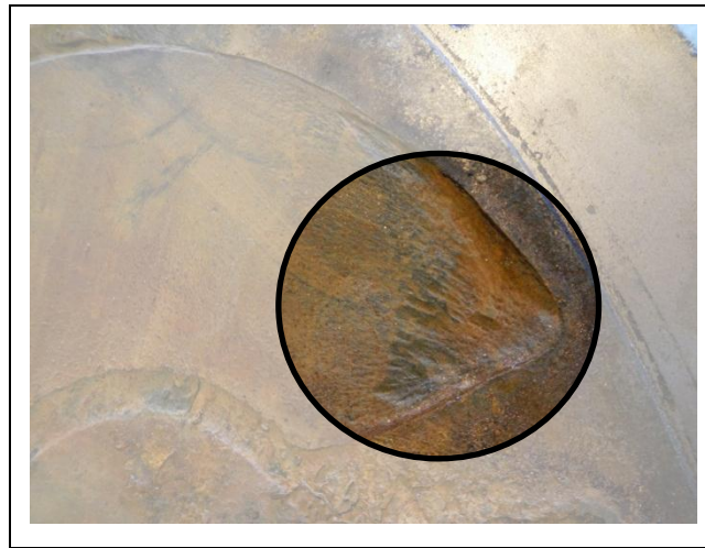
Figure 29: Sign of cavitation on casing
