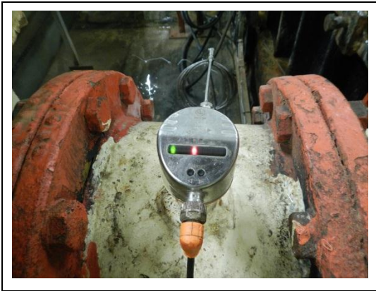
Figure B-15: Suction flow switch
