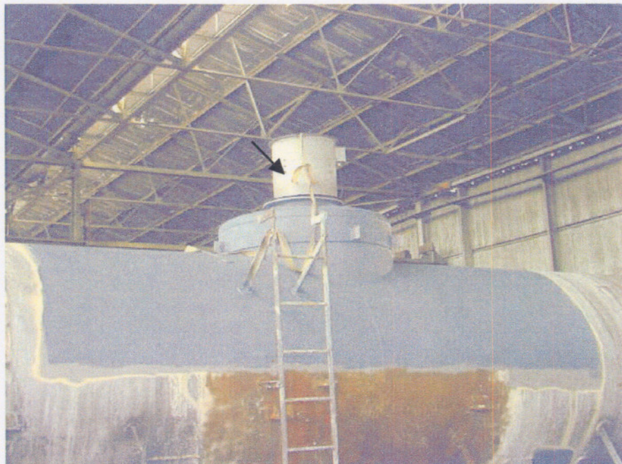
Figure 3.12: Ventilation fitting (extraction fan), which is mounted at the top opening of the tanker
