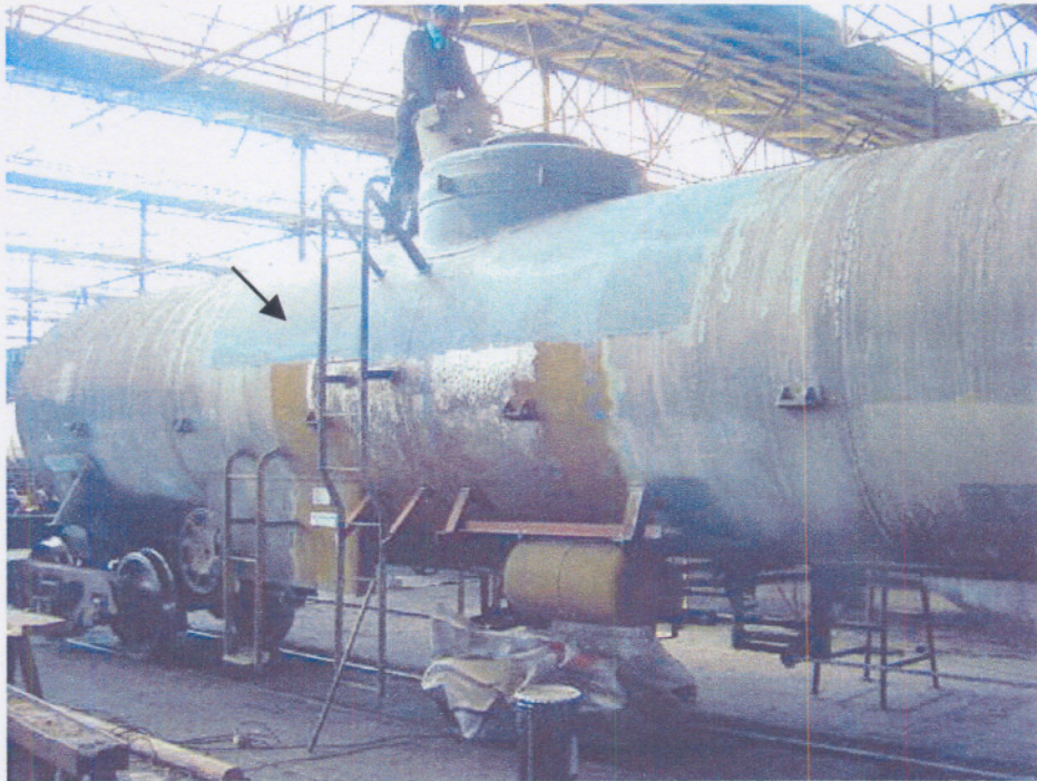
Figure 3.9: A close-up view of the grey area, which indicates the workspace for the dome area work process
