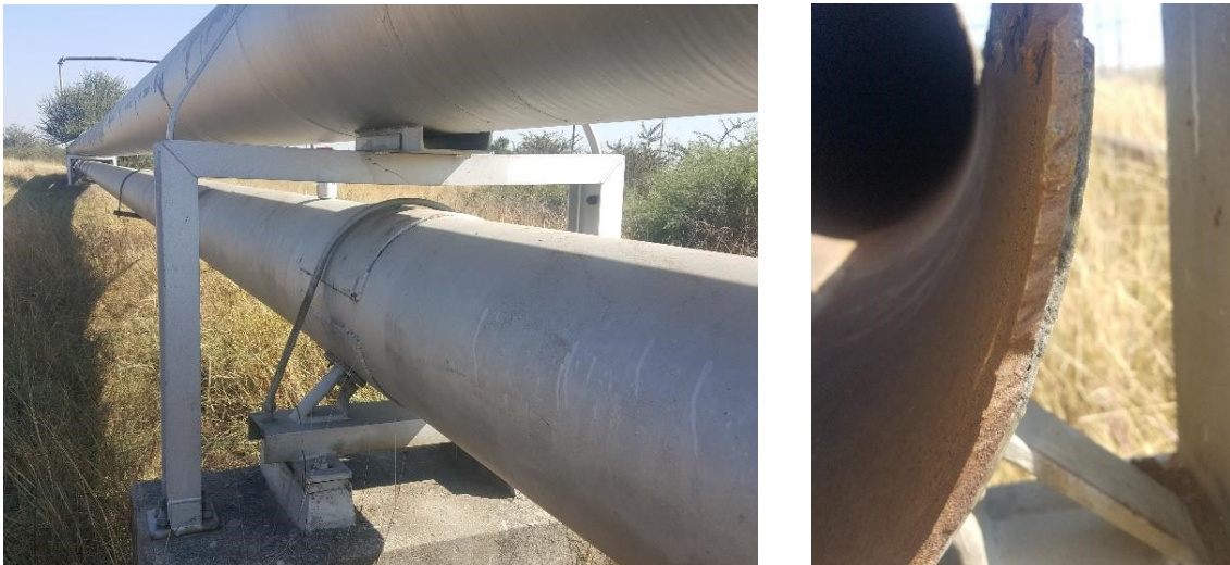
Figure 13 - Standard galvanised compressed air distribution pipes 2
