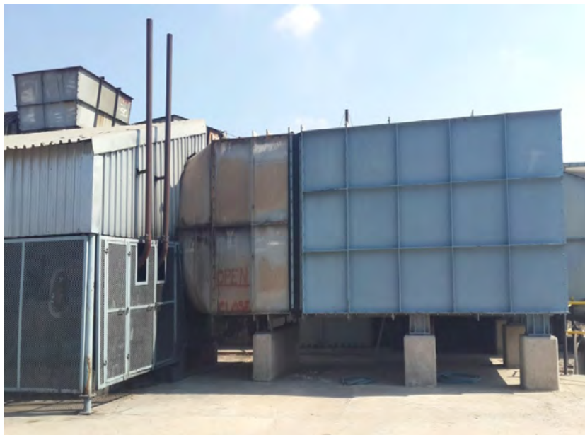
Figure 24: Main ventilation fans of mine A.
