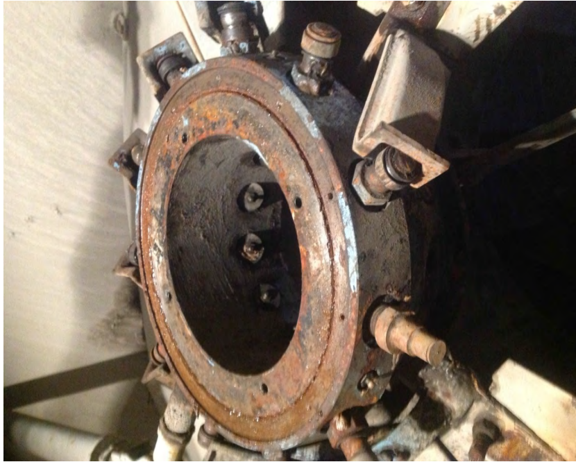
Figure 26: Failure in IGV Hub
