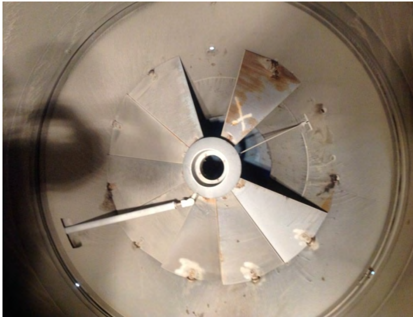
Figure 25: Typical IGV failure.
