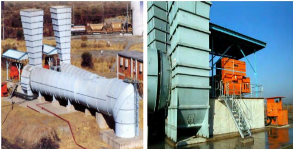
Figure 11: Typical mine ventilation fans [35].
