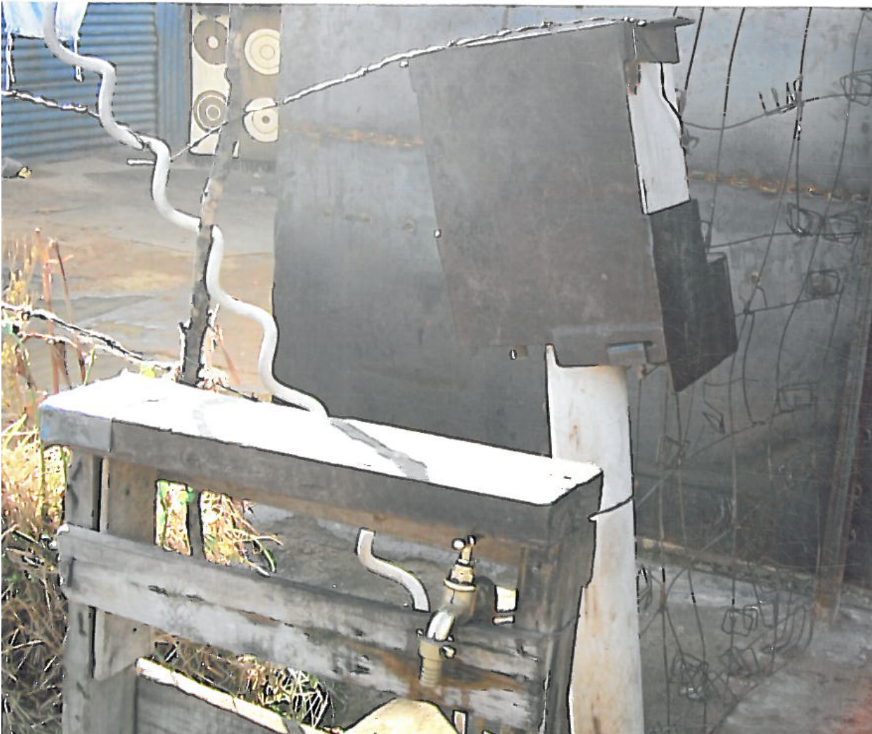
Illustration 5: A prepaid meter box and a tap installed by ELM. (Photograph: CT Musa).
