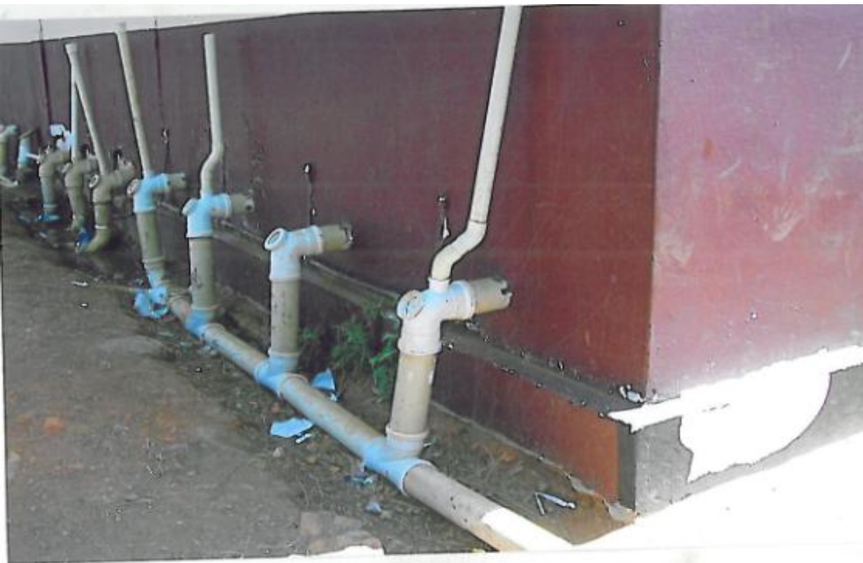
Illustration 7: Conventional flush toilets at Boiketlong Christian Primary School. (Photograph: CT Musa).
