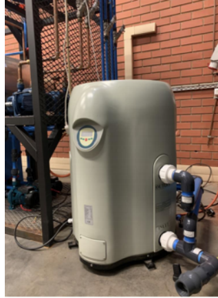
Figure 4.6: Heat pump used in heated two-tank plant
