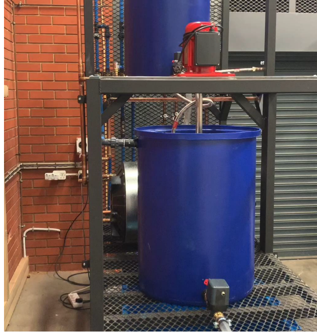
Figure 4.8: Agitator installed to ensure uniform heat distribution
