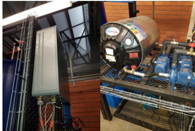
Figure 4.7: Gas heater used for heating of water in the system
