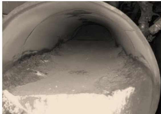
FIGURE 2.15: PRESENTATION OF SEVERE PC SETTLING INSIDE A PA TUBE (MODIFIED AFTER VAN DER MERWE, 2014)
