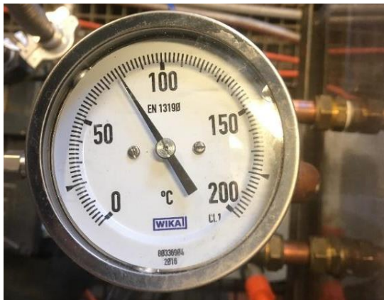
Figure 3-17: Temperature gauge displaying the temperature of steam entering the evaporation chamber inside the heat exchange piping
