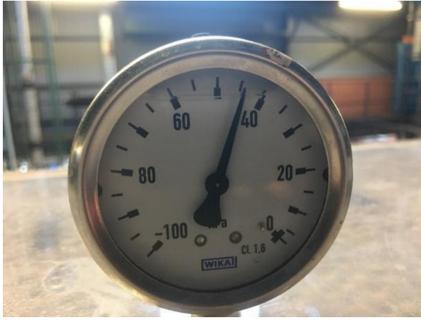
Figure 3-18: Vacuum gauge displaying vacuum inside evaporation chamber
