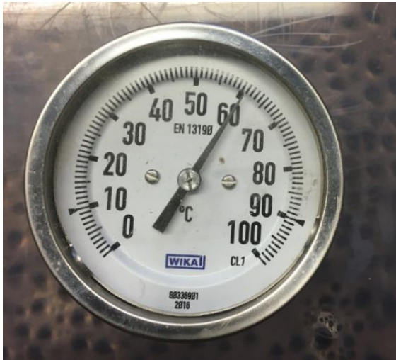
Figure 3-19: Temperature gauge displaying temperature inside evaporation chamber
