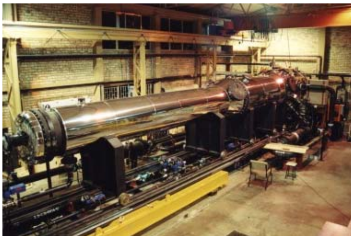
Figure 6.5: Completed PBMM plant
