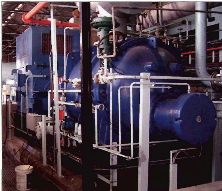
Figure 41 - Howden refrigeration machine
