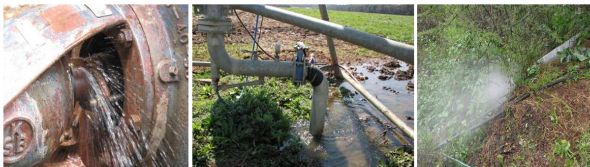
Figure 7-6: a) Leaking pump seals, b) Leaking main line, c) Rusted and leaking main line.
