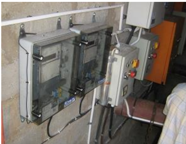
Figure 9: Meter before burn-out
