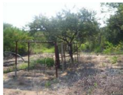
Figure 4: Pump station in the open veldt
