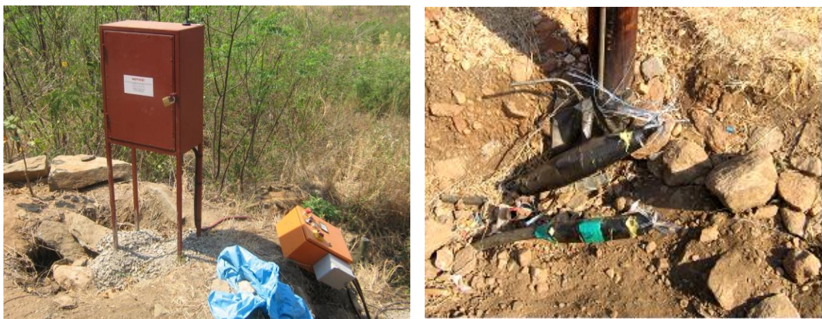
Figure 6-6: Pump station consisting only of DBs in the open veldt, b) Cable theft.
