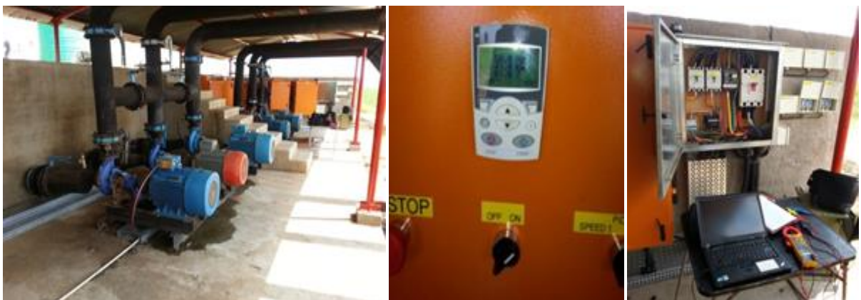
Figure 4-9: (a) Pump station with 6 pumps, (b) VSD controller, (c) Equipment setup.
