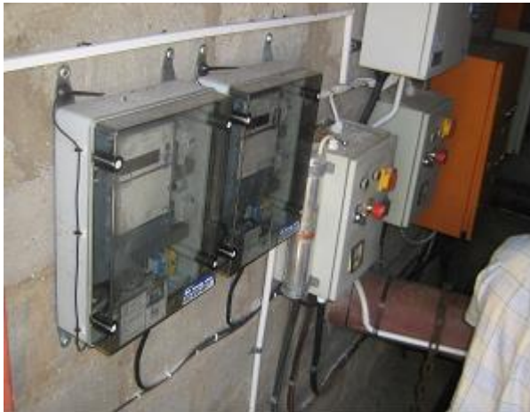
Figure 9: Meter before burn-out
