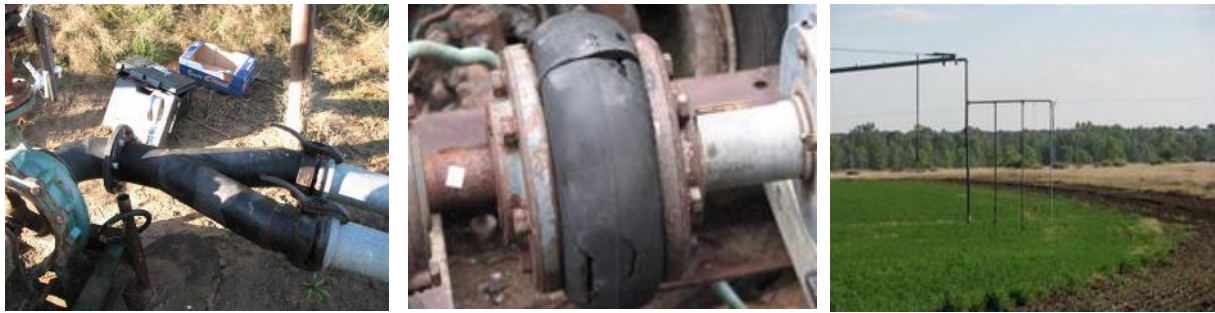
Figure 4-3: a) Incorrect suction fitting, b) Damaged Fenner Coupling, c) Inefficient pivot extension.
