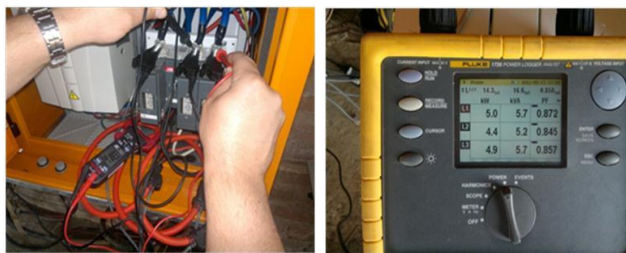
Figure 5: (a) Measurements done by M&V with a calibrated handheld meter. (b) Fluke power meter-measurements compared with M&V meter.
