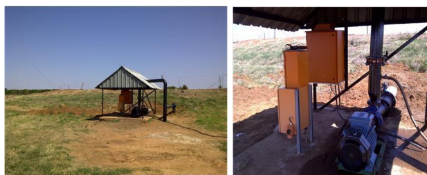
Figure 9: (a) Pump Station E4 visited by M&V Team. (b) VSD enclosure, new pump motor and Elster meter.
