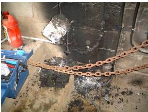
Figure 10: Wall burnt where meters was located
