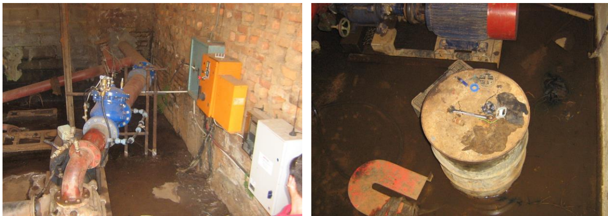
Figure 6-4: a) Inside a pump station showing piping, the control DBs and water on the floor, b) Pump station floor covered with water with a metal drum the only dry place to stand.
