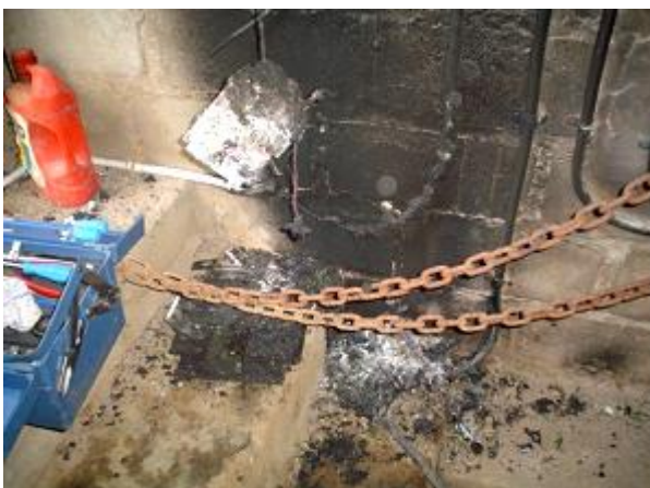
Figure 10: Wall burnt where meters was located
