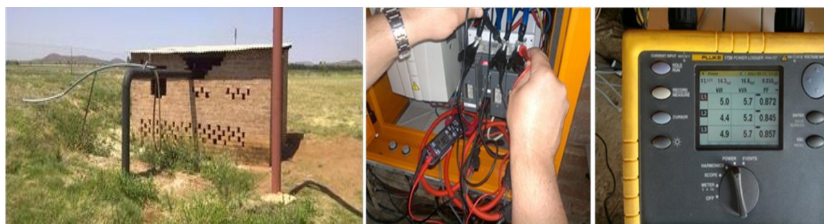
Figure 4-6: (a) Pump station 1, (b) Measurements done by M&V with a calibrated handheld meter, (c) Fluke power meter - measurements compared with M&V meter.
