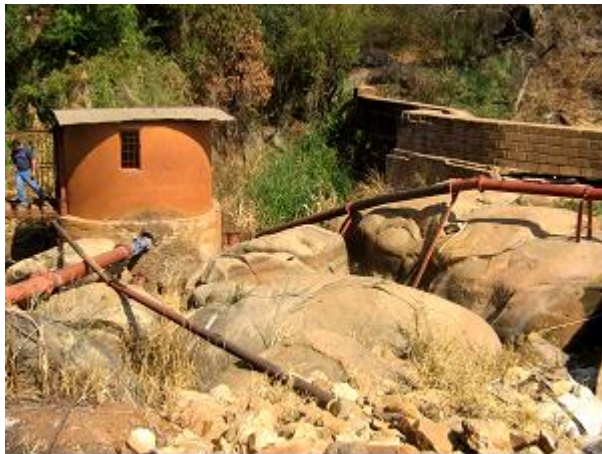
Figure 3: Pump station at the river
