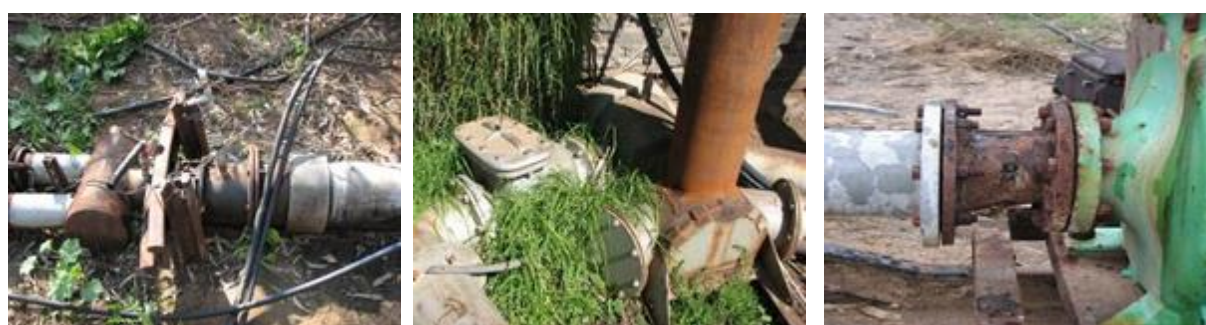
Figure 4-2: a) Restrictive Manifold, b) Pipe bends and manifold, c) Incorrect eccentric fitting.
