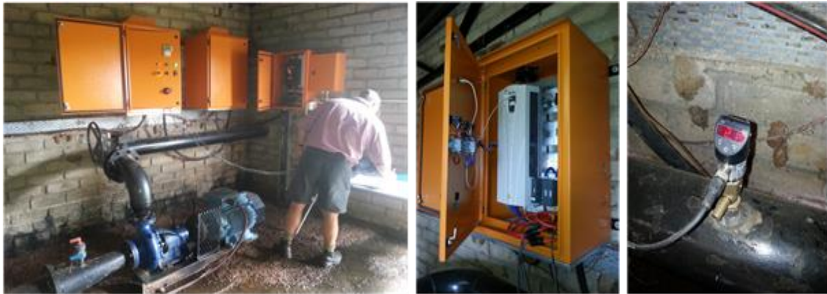
Figure 4-8: (a) Inside irrigation pump station, (b) VSD in enclosure, (c) Water line pressure transducer.
