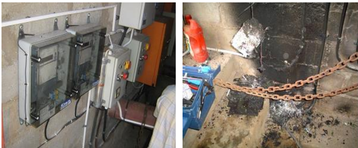
Figure 6-7: a) Three phase power meter installation, b) Meter burnt-out due to failed PF capacitor.
