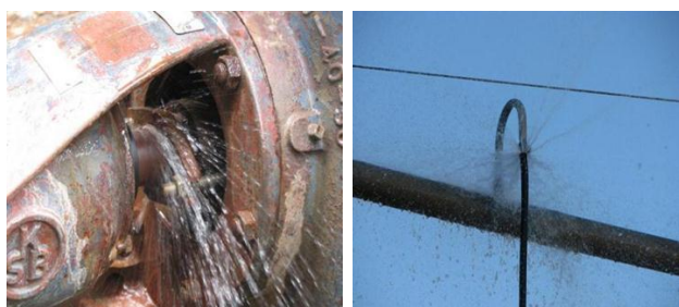
Figure 1: (a) Leaking pump seals. (b) Leaking sprinkler tubes. [4]
