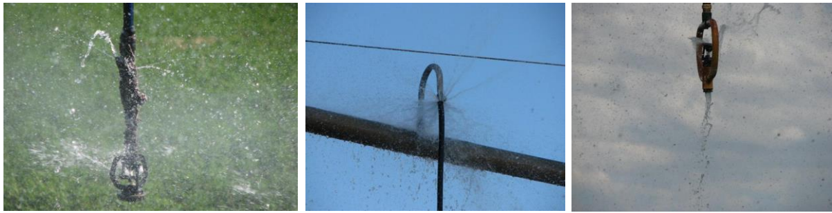
Figure 7-7: a) Burst nozzle tube, b) Leaking sprinkler tubes, c) Leaking nozzle.
