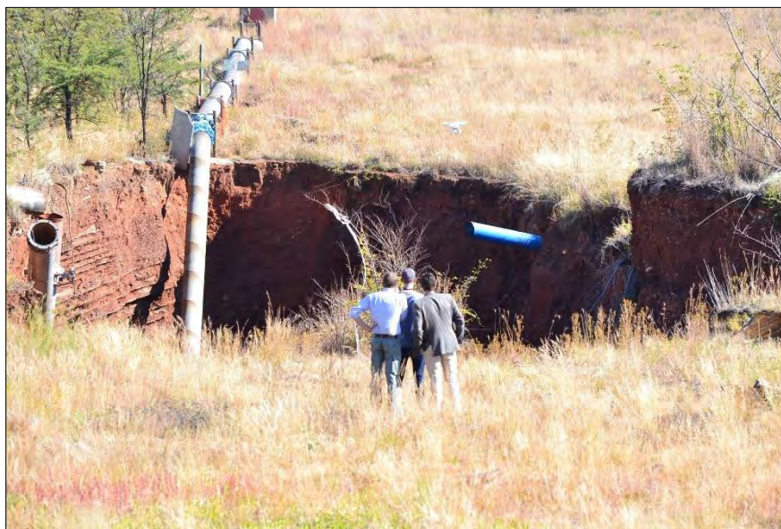
Figure 2-1: Sinkhole at Carletonville reservoirs
