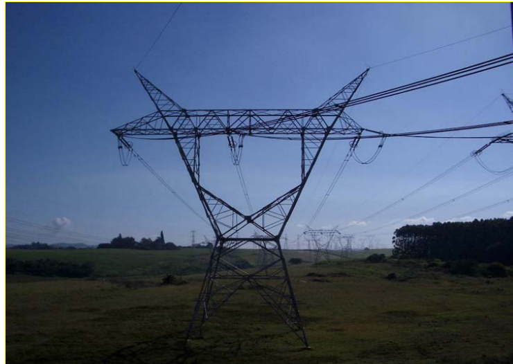
Figure 5.10: Tower 1 near Athene substation [15]
