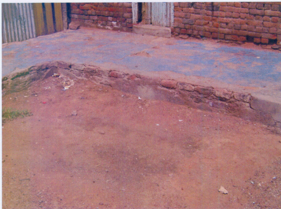
Figure 5: Contaminated building in Prieska. (See blue asbestos in foundation)
