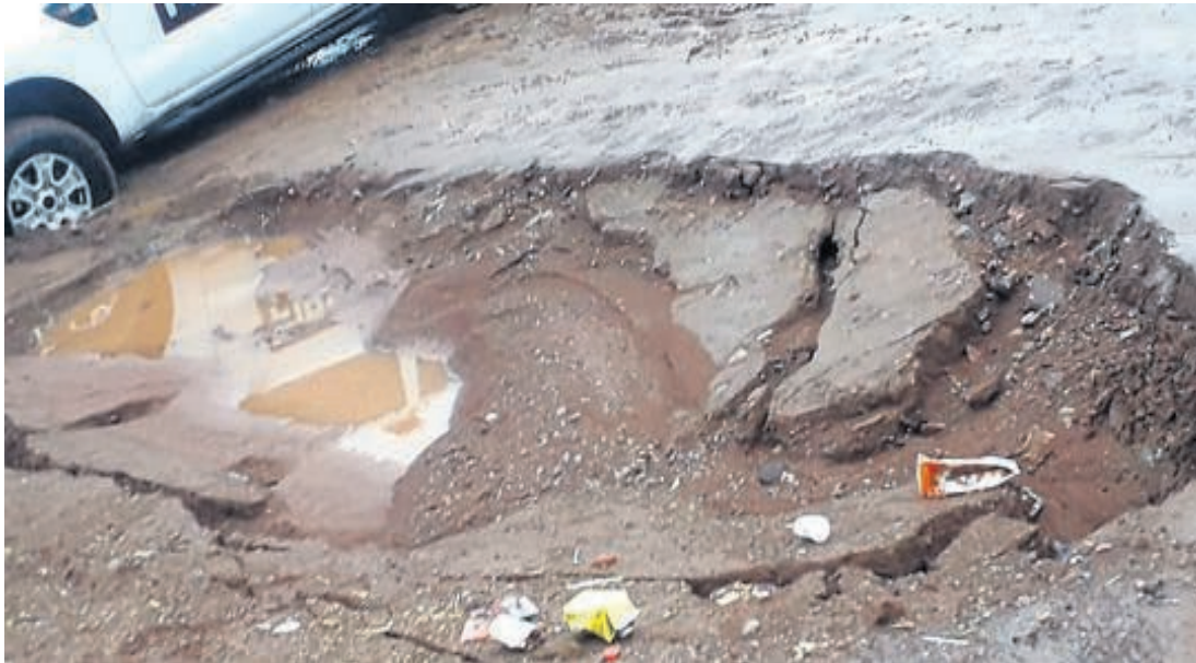
Figure 49 Rain Damaged Roads in Bekkersdal
