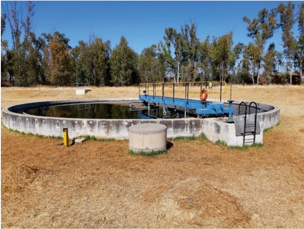
Figure 3-2: Recycled Activated Sludge (RAS) dam.
