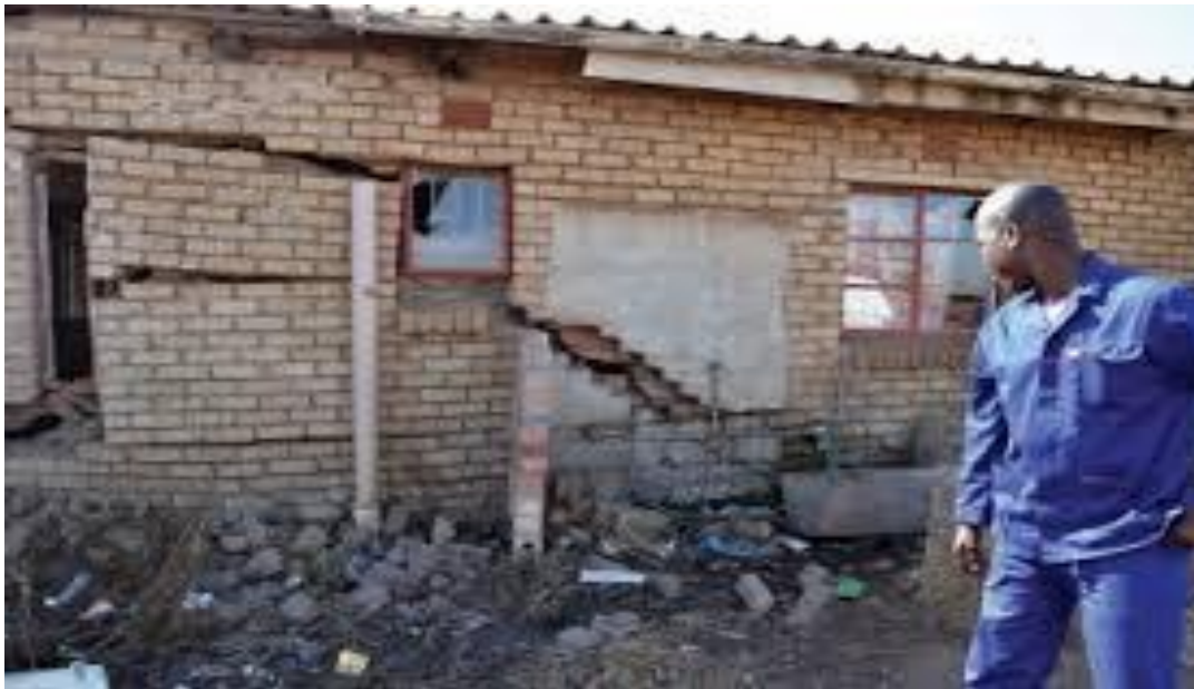
Figure 3.3 House cracks resulting from vibrations in mining in the West Rand District Gauteng. Source: (Herald, 2011).
