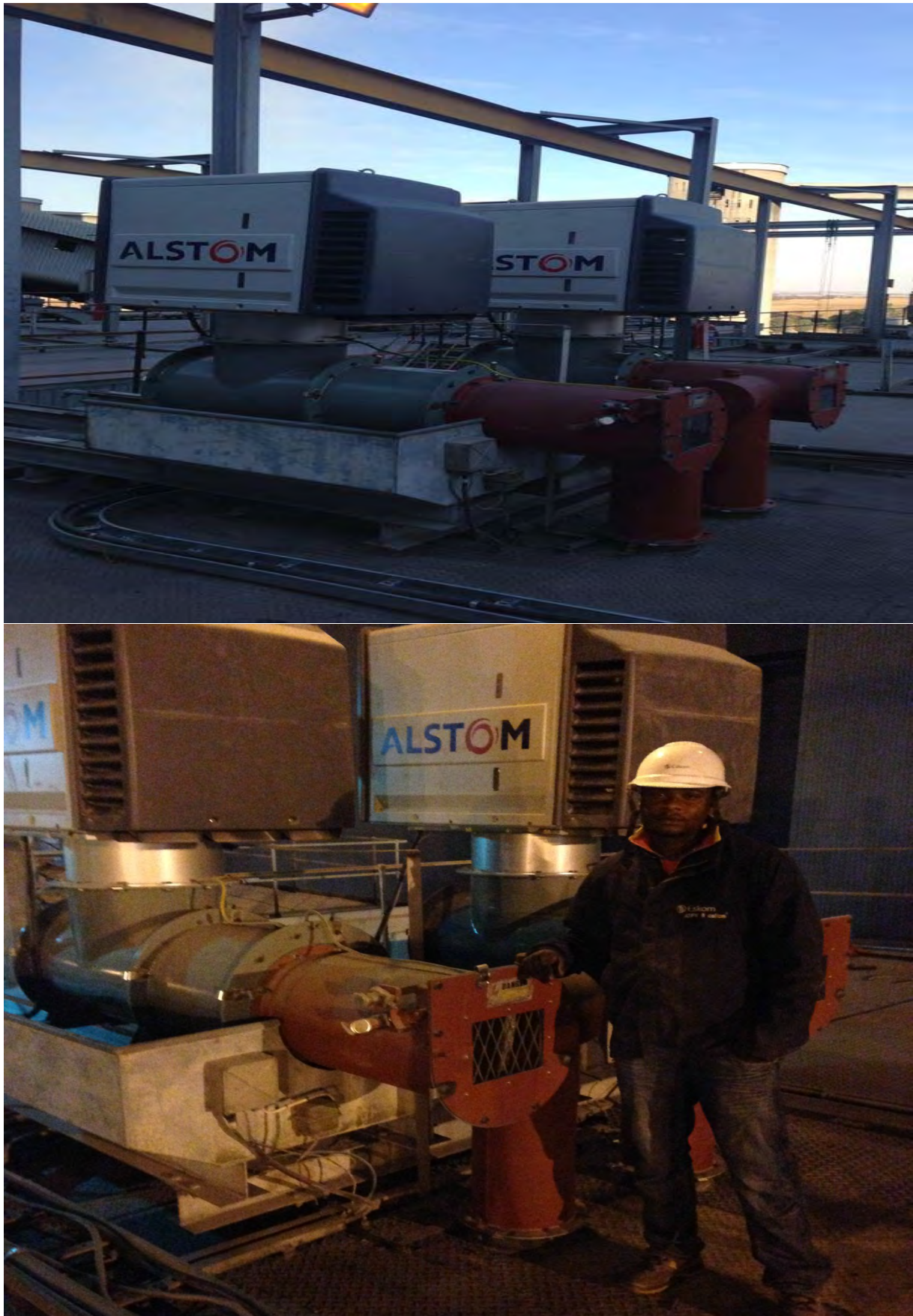
Figure 8-16: Installed and commissioned HFPS transformers
