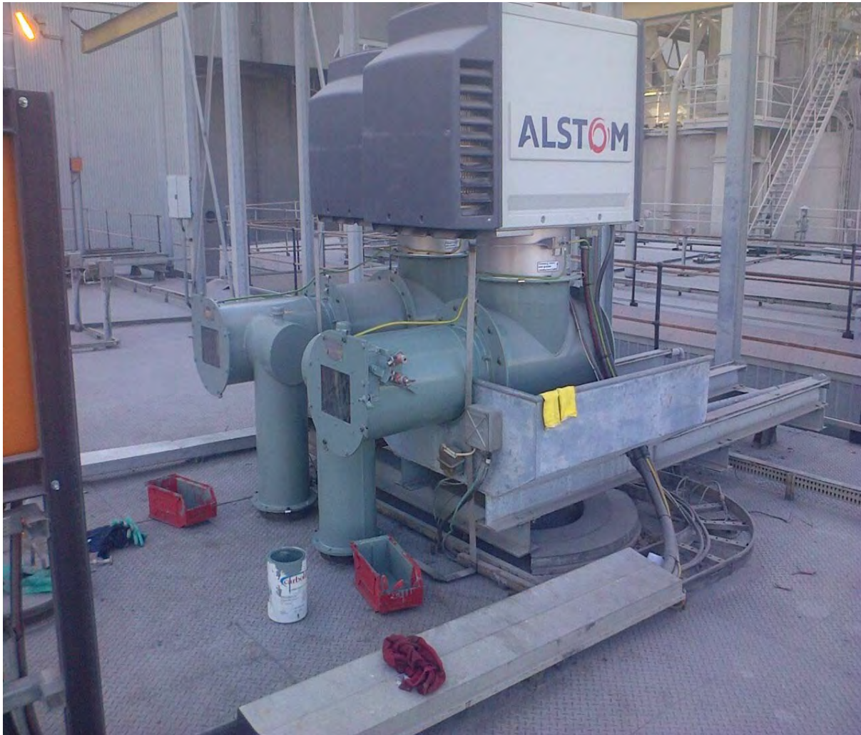
Figure 8-15: Installed HFPS transformers
