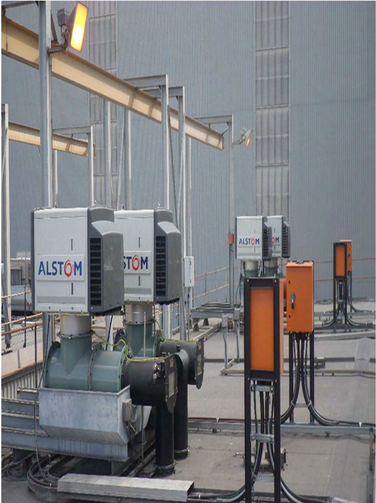
Figure 8-17: Fully commissioned HFPS transformers on the first four fields of an ESP casing
