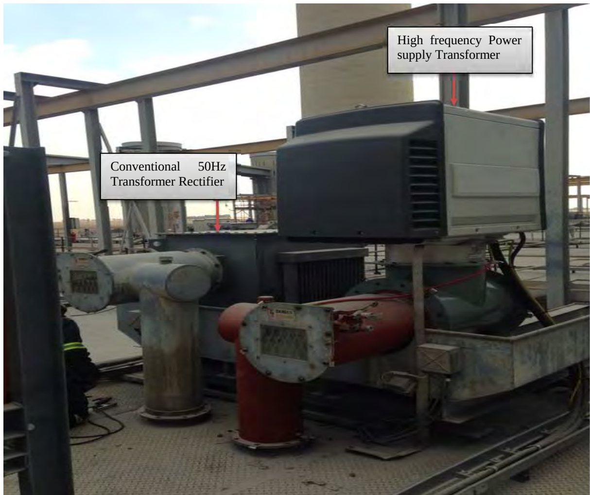
Figure 4-14: Conventional TR set and an HFPS transformer as installed in the plant
