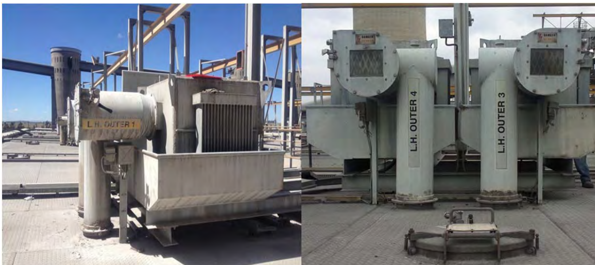
Figure 4-9: TR sets installed on an ESP field
