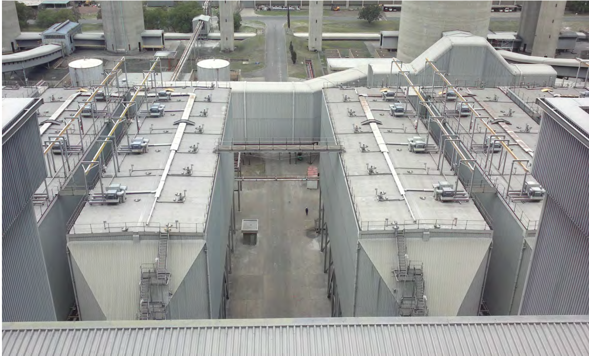
Figure 8-3: Largest electrostatic precipitator plant in Africa
