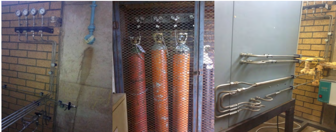
Figure 4-5: Gas cylinder and piping into the test oven
