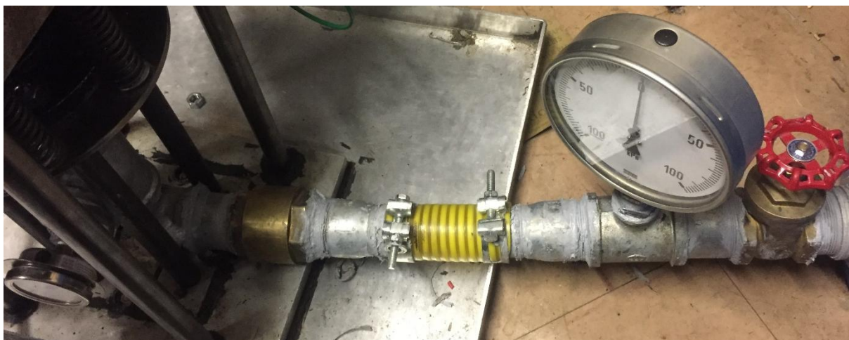
Figure 3-13: Inlet/suction pressure gauge, one-way valve, and gate valve
