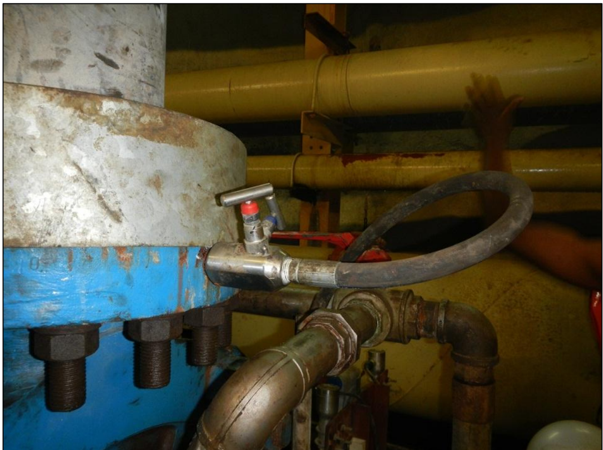
Figure 18: Discharge pressure transmitter
