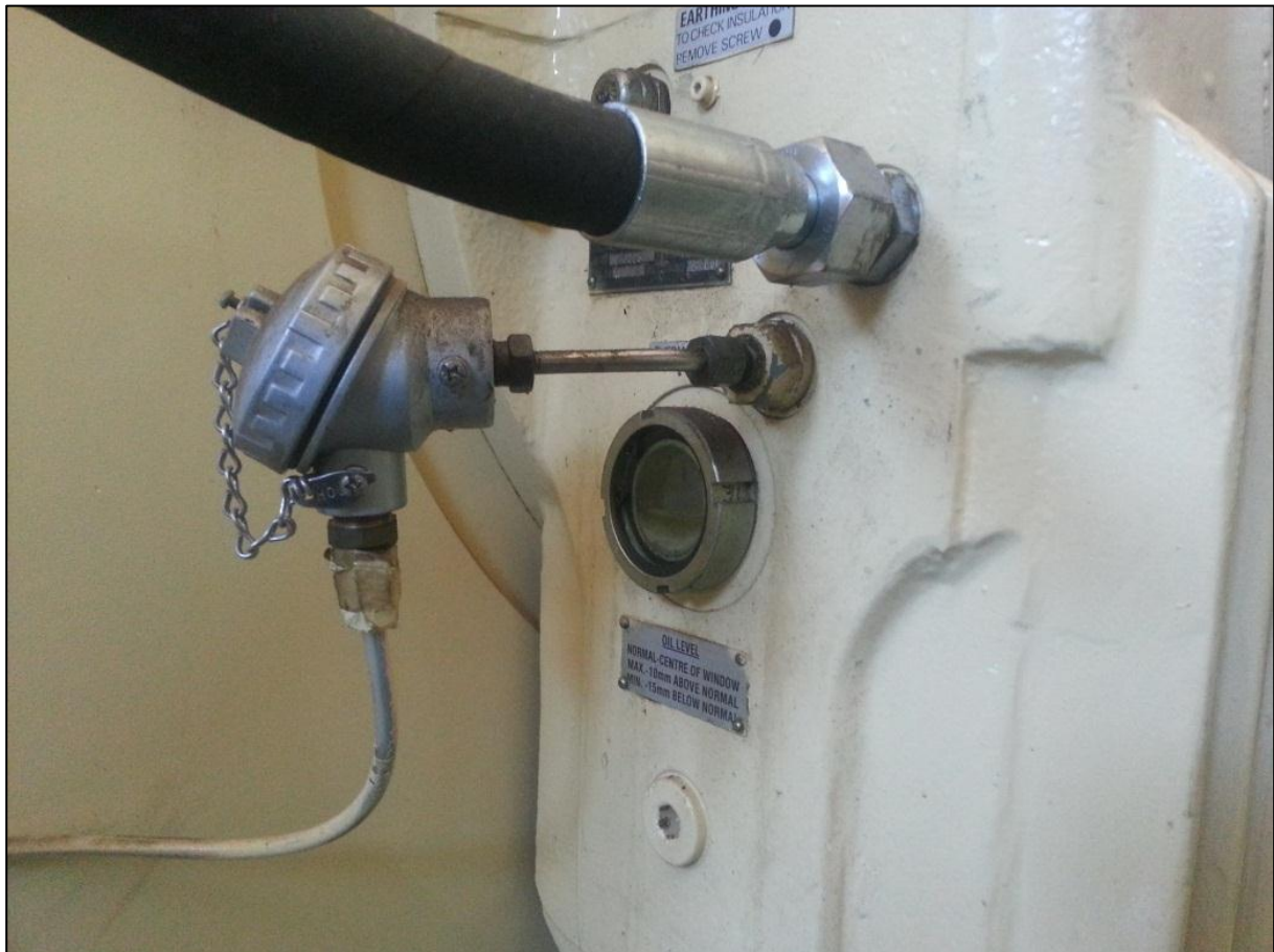
Figure 16: Temperature probe installed at the DE of motor
