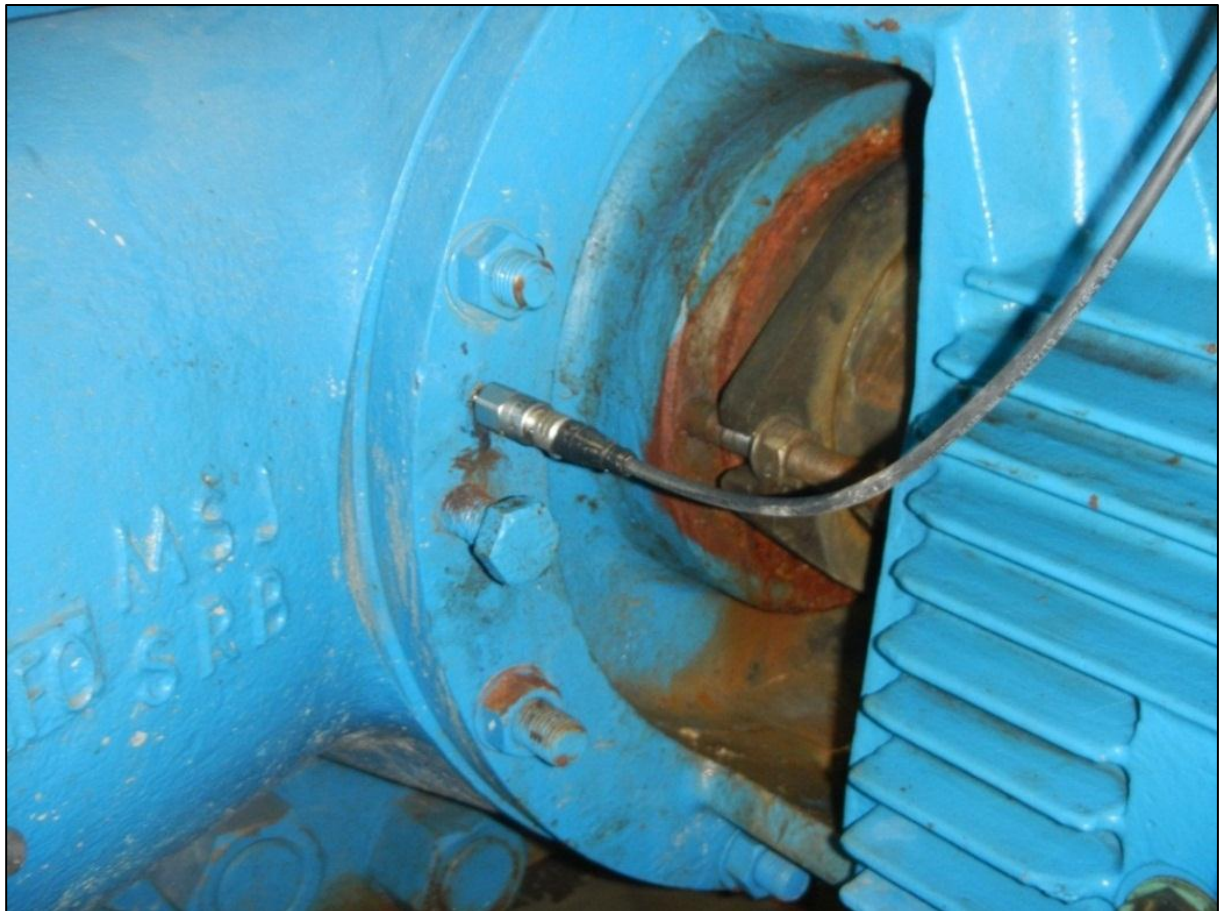
Figure 15: Vibration transmitter installed on the DE of the pump
