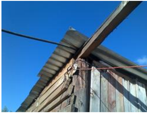
Figure 46: Informal electricity lines enter an informal backyard dwelling
