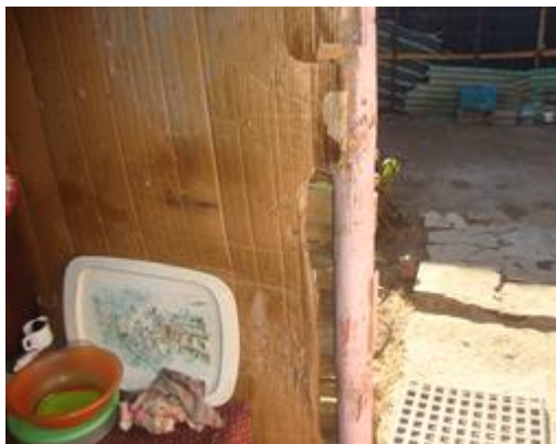
Figure 42: The inside of an informal backyard structure poorly insulated with cardboard
