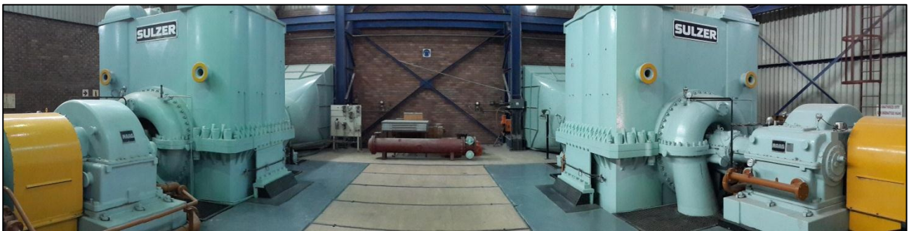
Figure 52: Multistage centrifugal compressors located at Mine A 21 .
