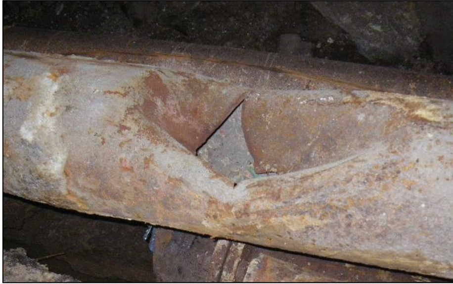
Figure 17: A leak found on a compressed air pipeline 10 .
