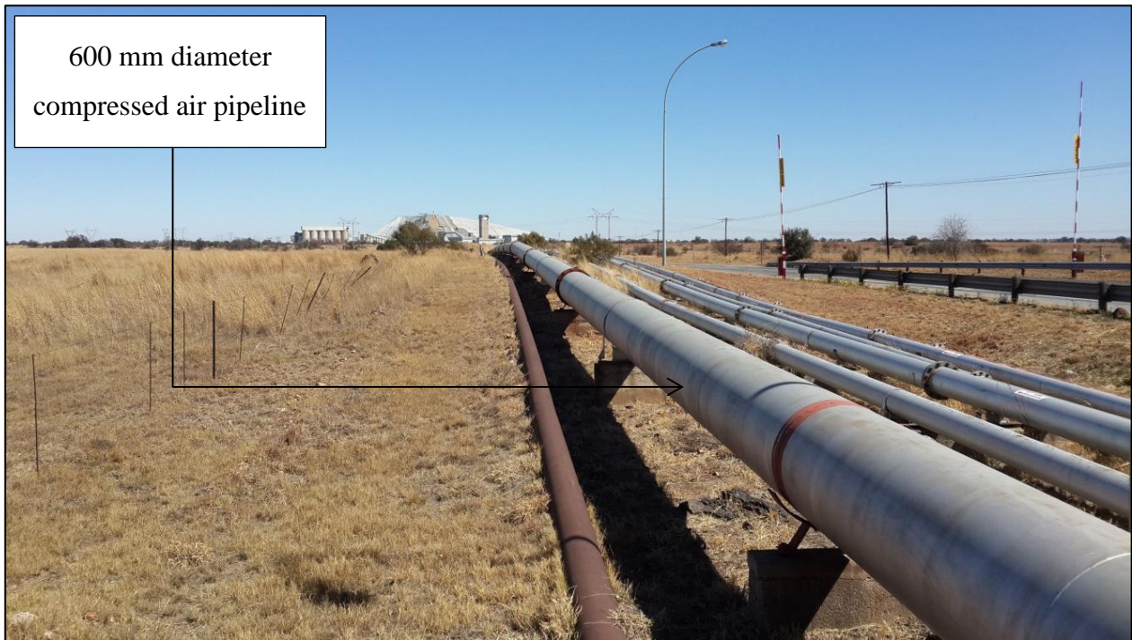
Figure 6: Steel pipe transporting compressed air to a mining shaft 4 .
