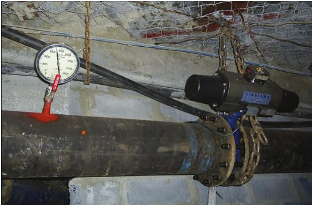
Figure 51: A butterfly valve and a pressure transmitter installed in a main pipeline.
